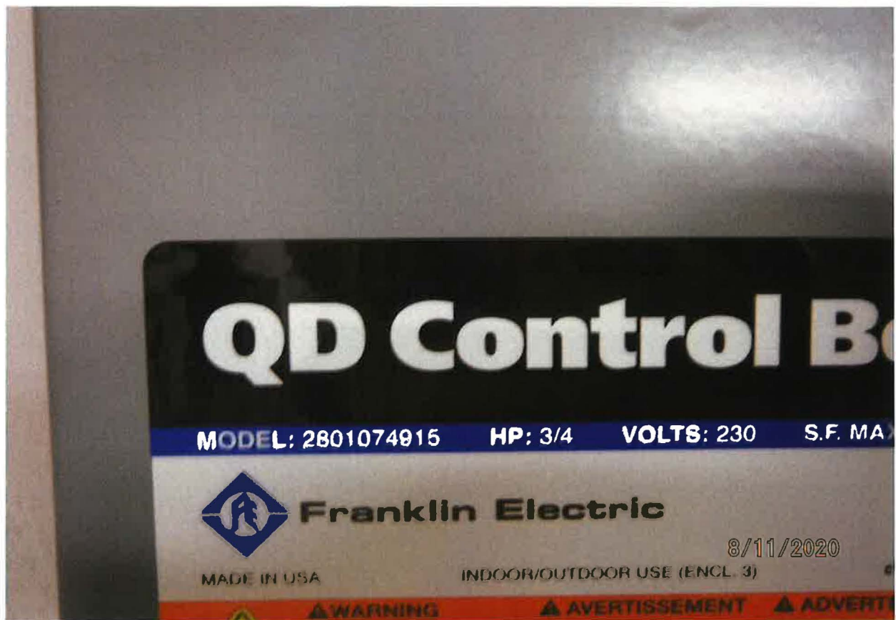
WELL No. 2 – ¾ HP PUMP
