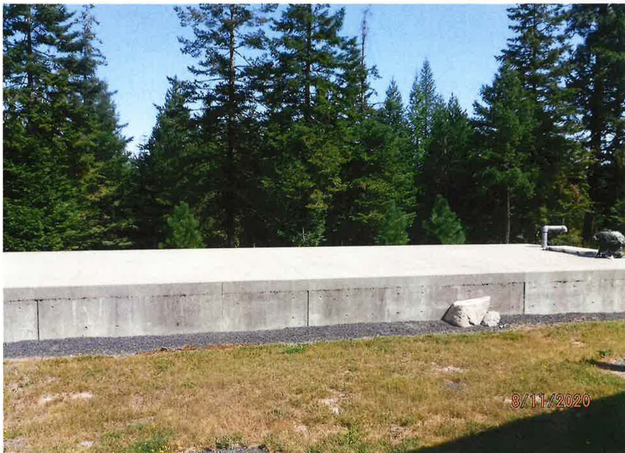
DOMESTIC & FIRE PROTECTION STORAGE - 72,145 GALLON STORAGE TANK
