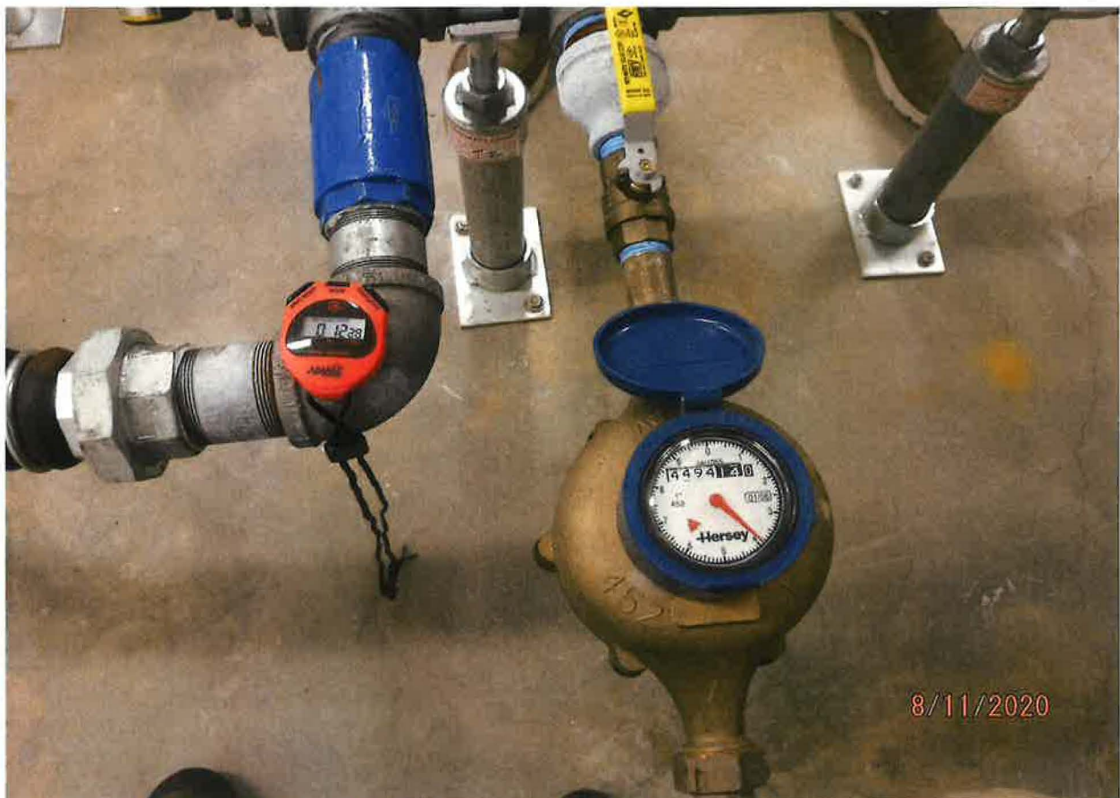
WELL No. 2 – MEASURING DEVICE
