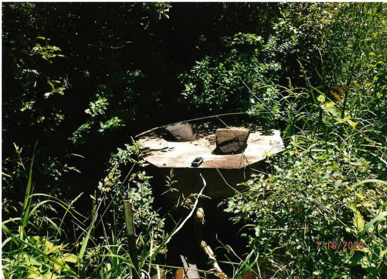
POD – 1 HP SUBMERSIBLE PUMP IN UNNAMED STREAM
