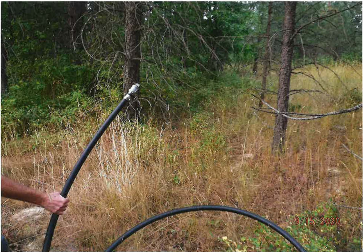
DOMESTIC POU – STUB IN PARCEL PIN: 0L0020010020; LT 2 BLK 1, ORCHARD SOUTH SUBDIVISION
