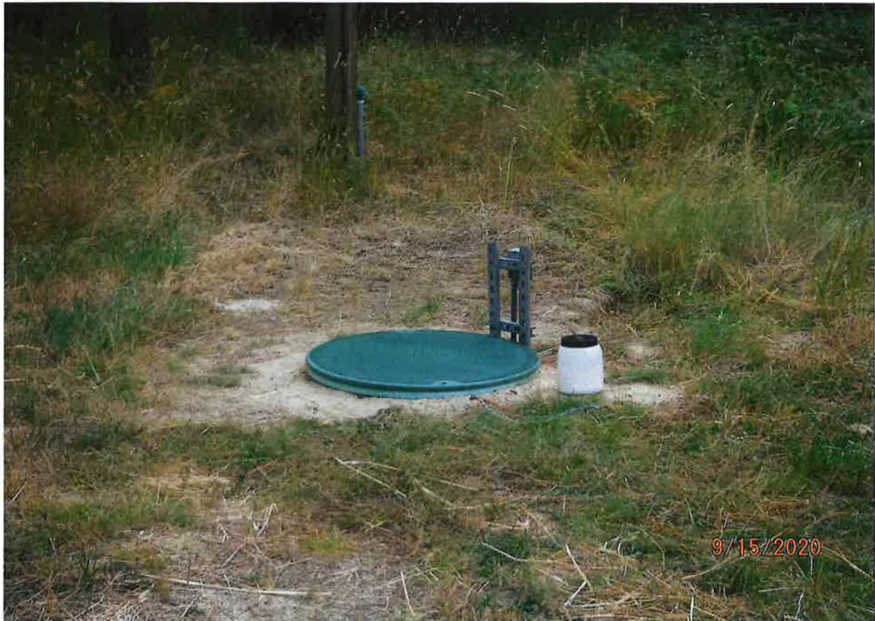
EACH DEVELOPED PARCEL HAS SEPARATE 3,000 GALLON STORAGE RESERVOIR
