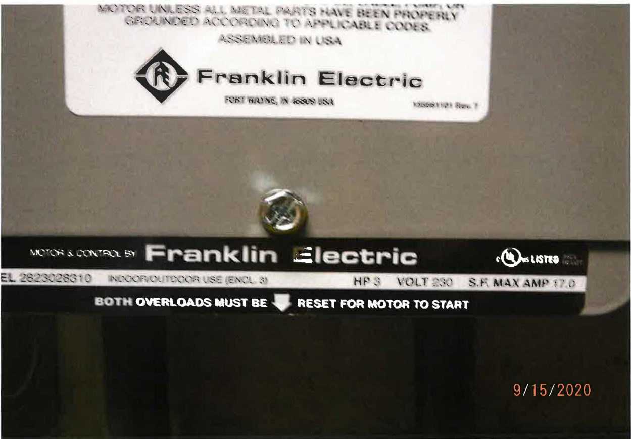
3 HP WELL PUMP
