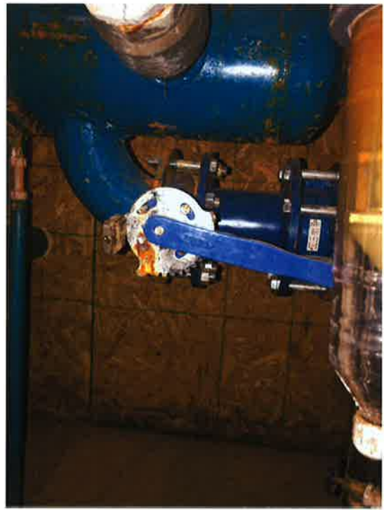
Photo #15 – Site Visit 10/20/2020 Valve that needs to be closed for the two well systems to be isolated.
