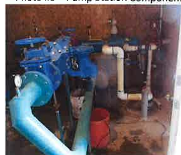
Photo #3 – Pump Station Components
