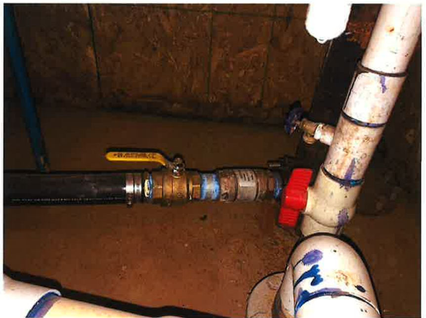
Photo #13 – Site Visit 10/20/2020 Small well was connected to black pipe that connects to the north side of the manifold.
