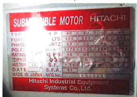
Photo #2 –40 HP Pump Information
