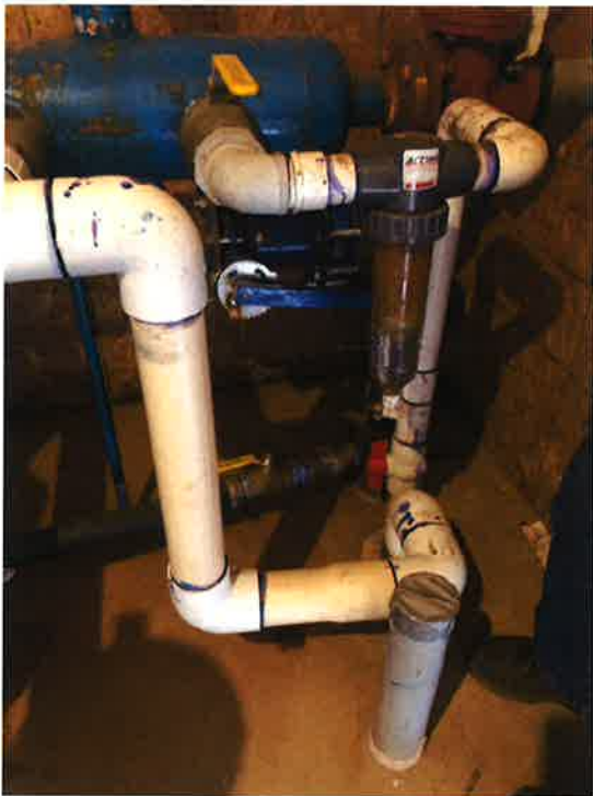
Photo #14 – Site Visit 10/20/2020 Updated water system on the north side of the manifold.
