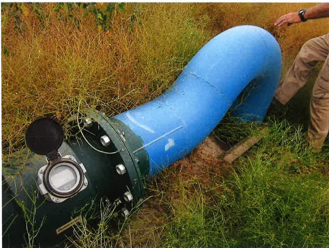
Figure 6: Injection well and meter
