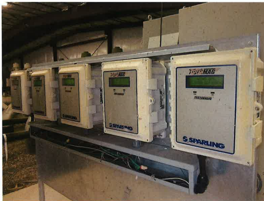
Figure 4: Readout displays for installed meters on pipelines
