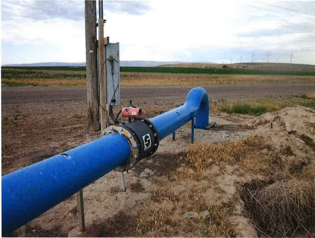
Figure 7: And another injection well with meter installed
