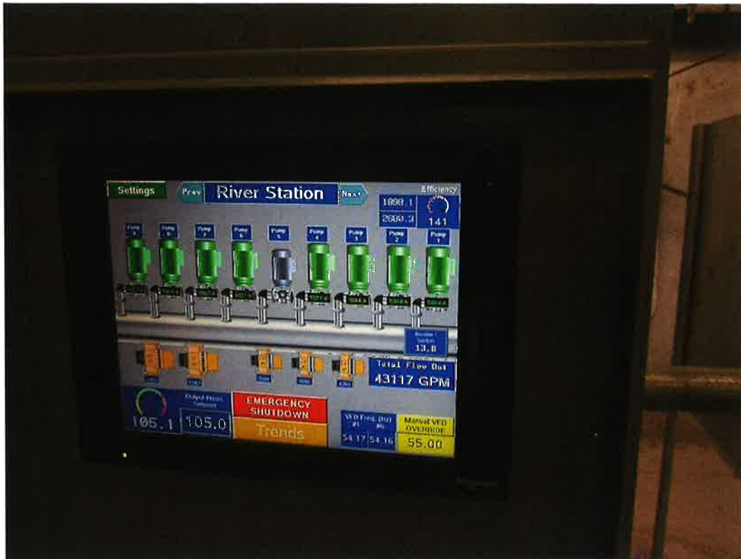
Figure 5: Pump station control
