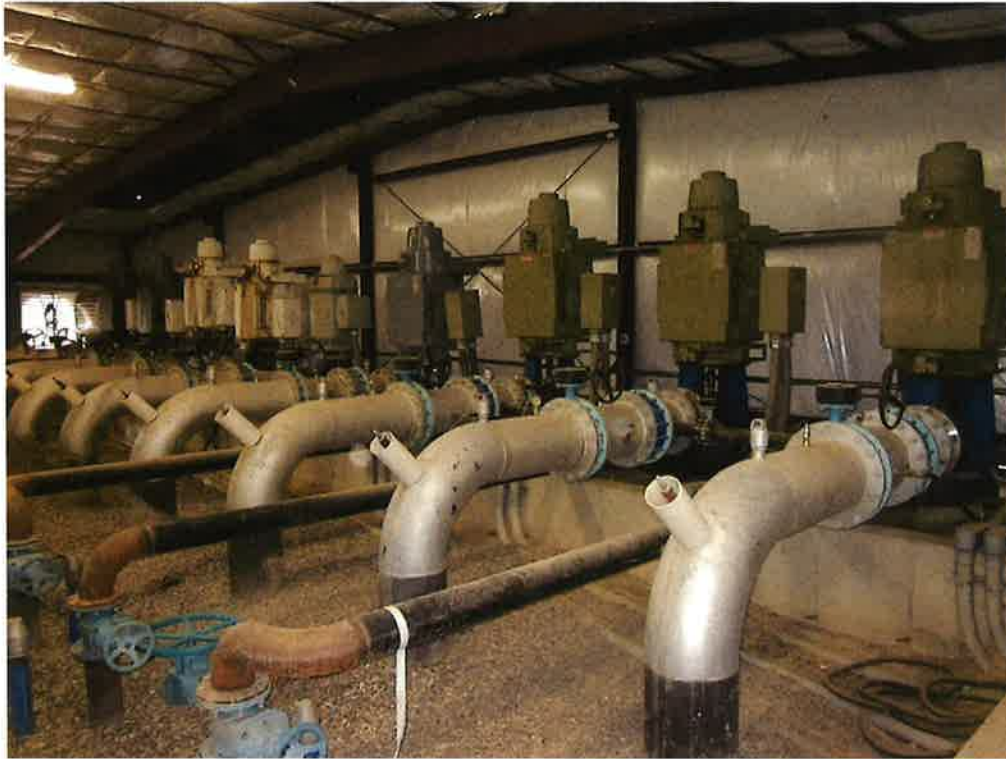
Figure 3: Pumps inside the pump station
