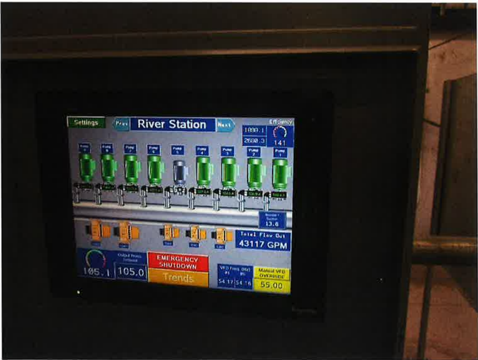
Figure 8: System control screen inside pump station
