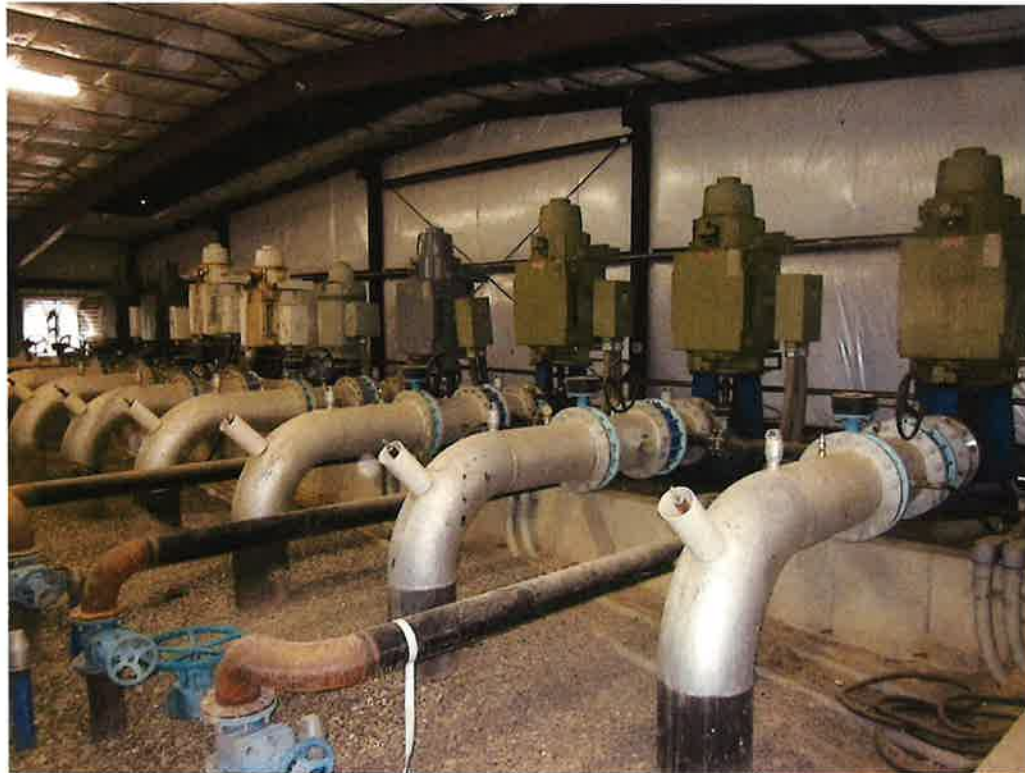
Figure 6: Pumps inside pump station
