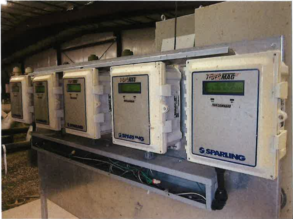
Figure 7: Meter displays inside pump station
