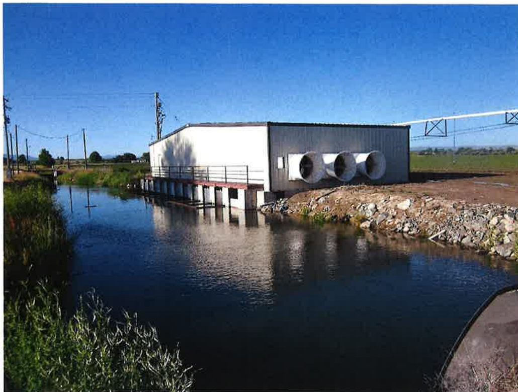
Figure 5: SWID pump station
