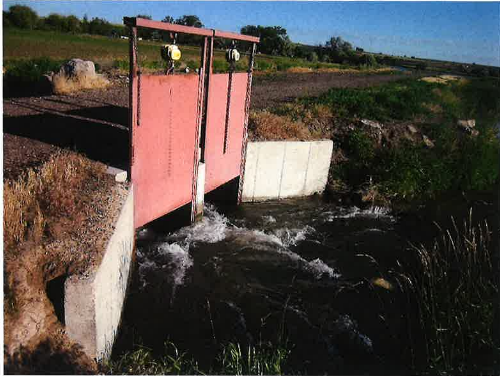
Figure 3: Headgate southwest side of wetland diverting into return canal
