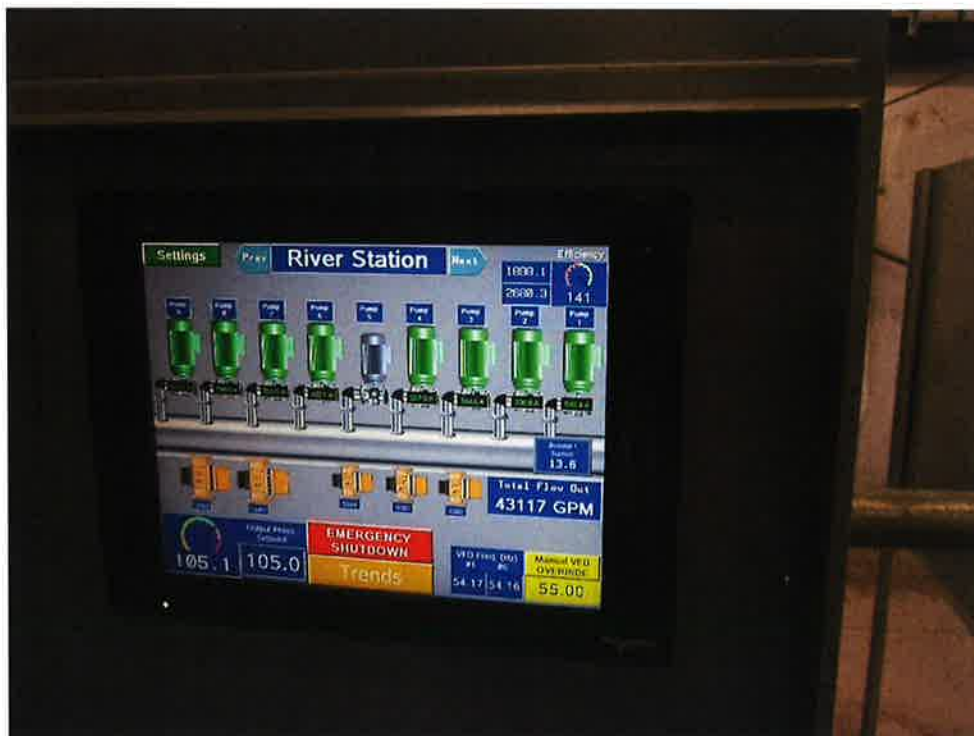
Figure 8: System control screen inside pump station
