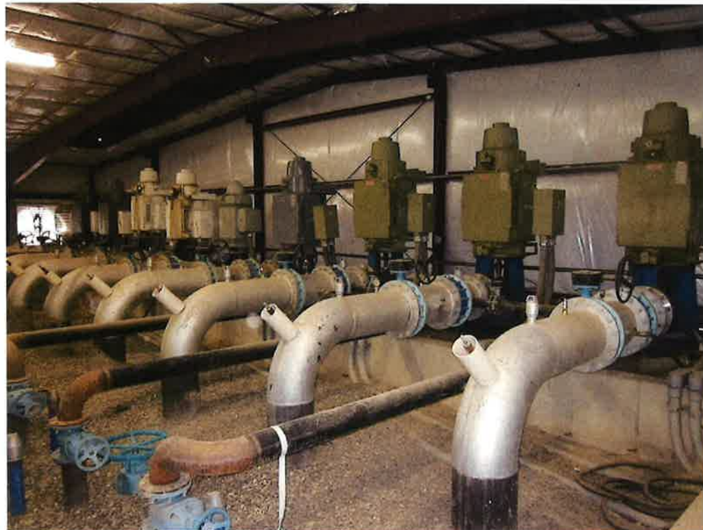
Figure 6: Pumps inside pump station
