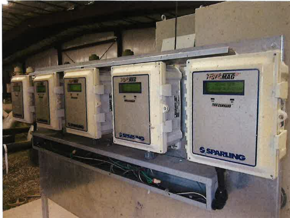
Figure 7: Meter displays inside pump station
