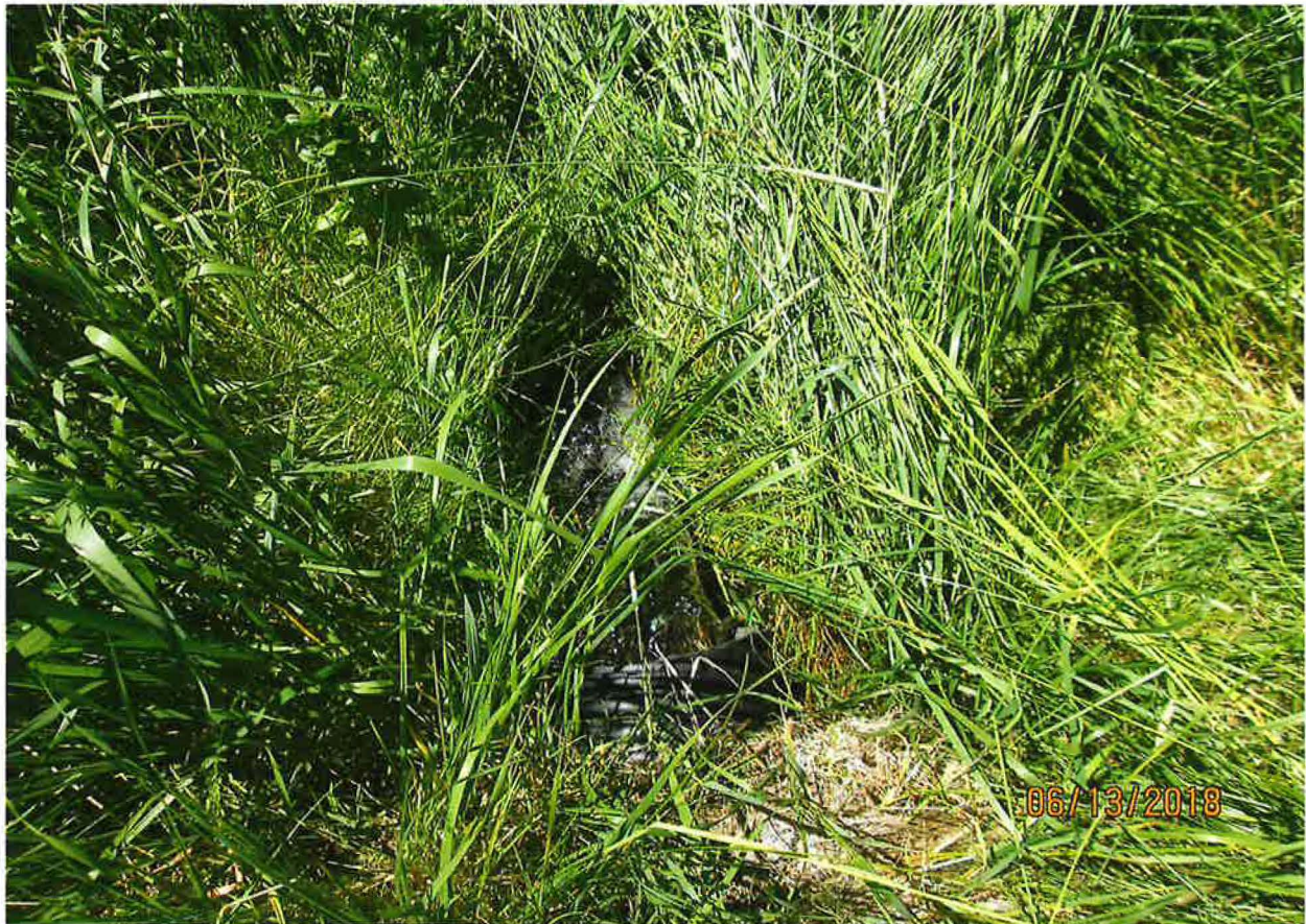
POND OVERFLOW DISCHARGE BACK TO STREAM VIA 6" CORRUGATED PVC PIPE
