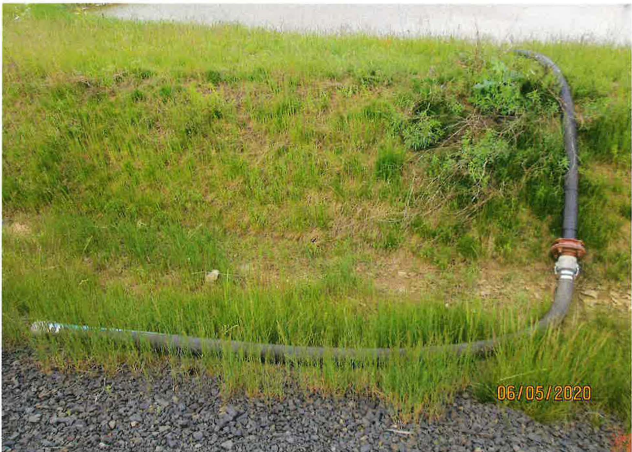
INDUSTRIAL FROM STORAGE PUMP FROM POND-TO-WATER TRUCK VIA HOSE CONNECTION
