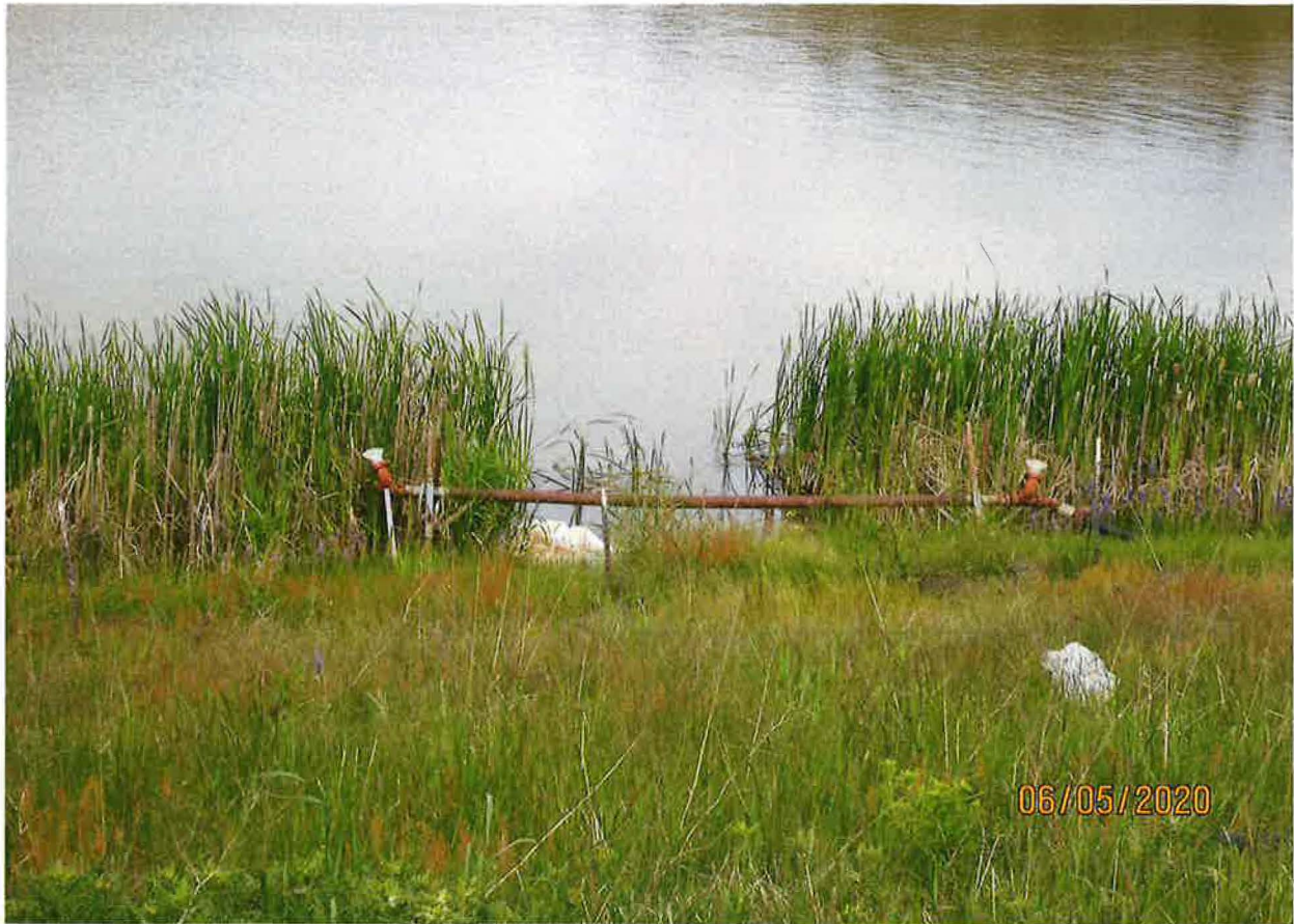
INDUSTRIAL FROM STORAGE POU - PUMP SYSTEM FROM POND TP1
