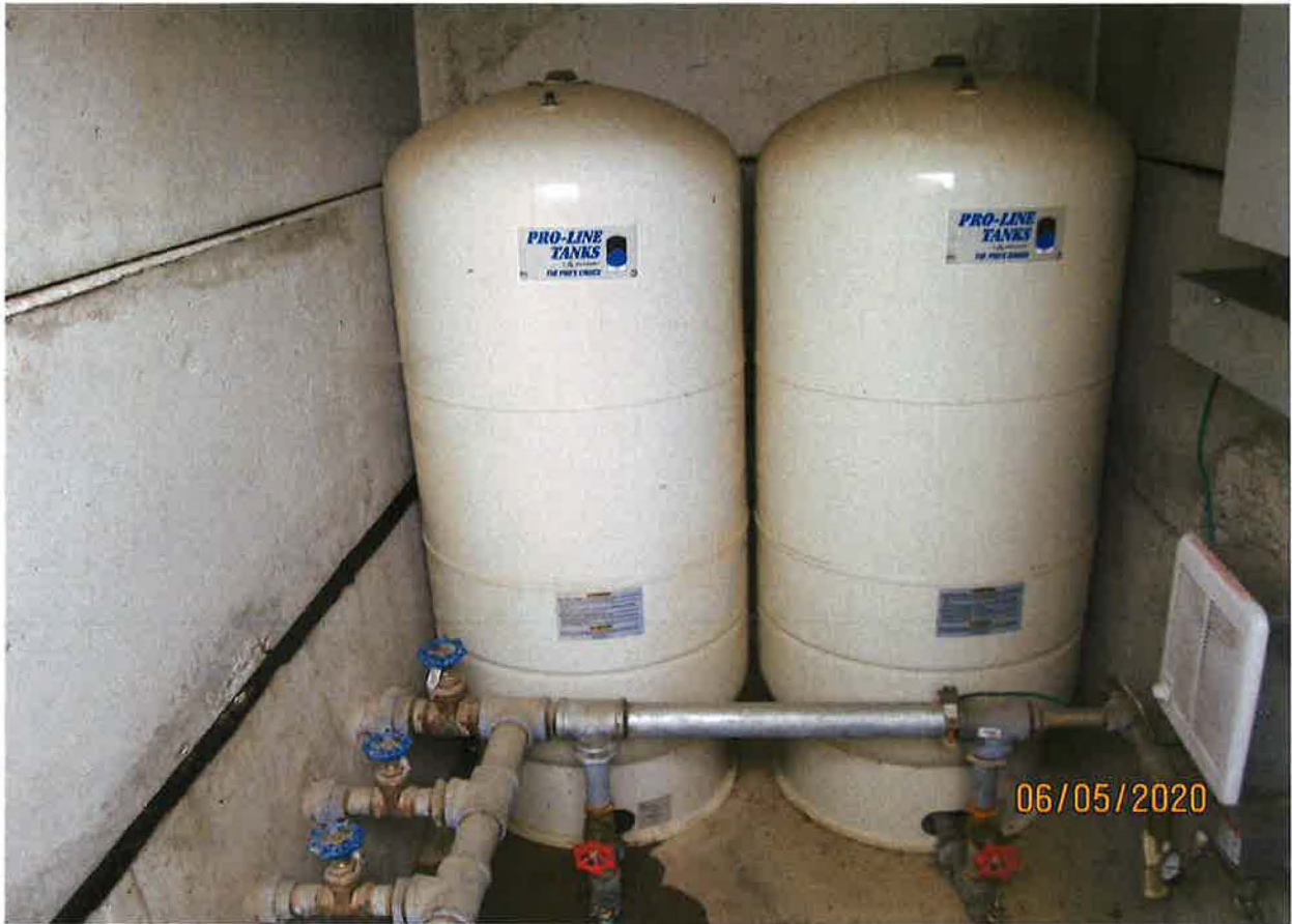
IRRIGATION WATER CONVEYANCE SYSTEM PIPING IN PUMP VAULT
