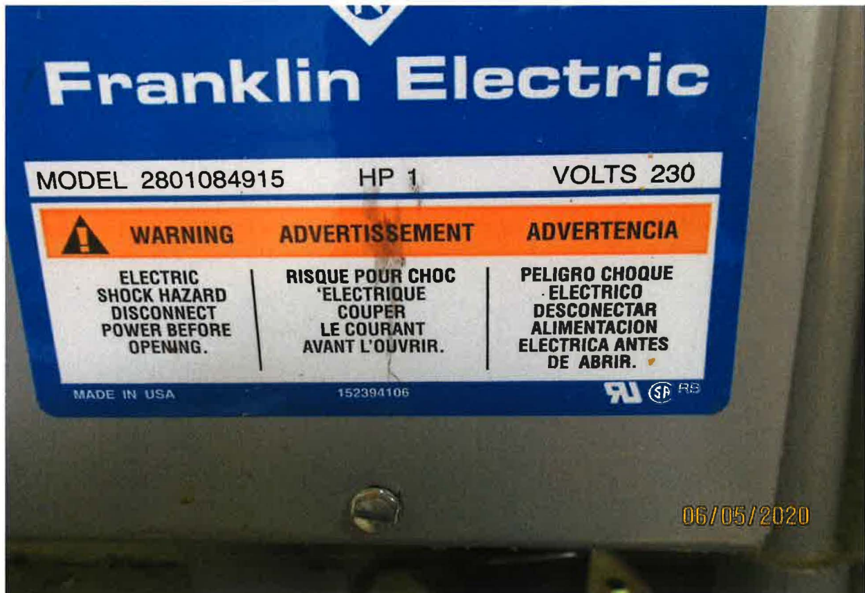
EACH STORAGE TANK HAS A 1HP DISTRIBUTION PUMP
