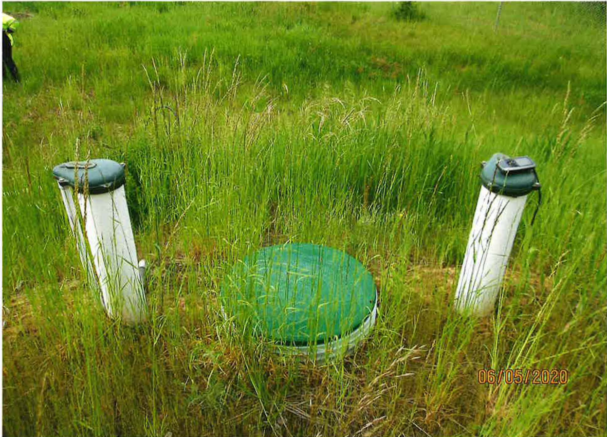
2EA 5,000 GAL STORAGE TANKS
