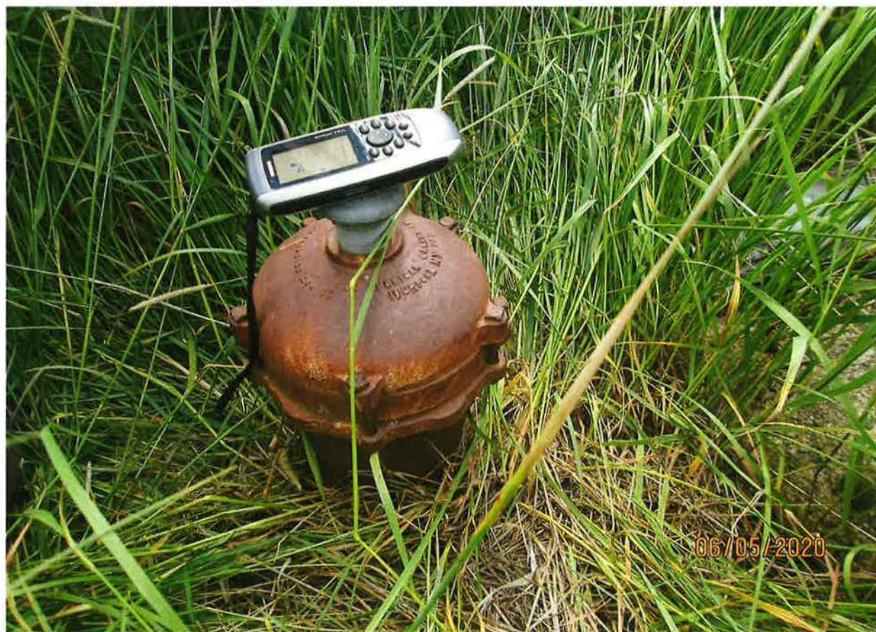
POD - WELL 95-90-N-32
