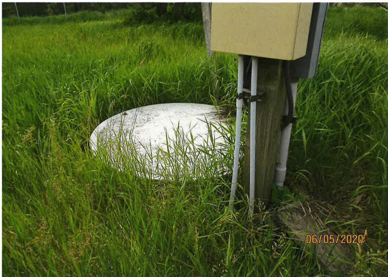
AT GROUNDWATER POD – WELL PUMP CONTROL PANEL
