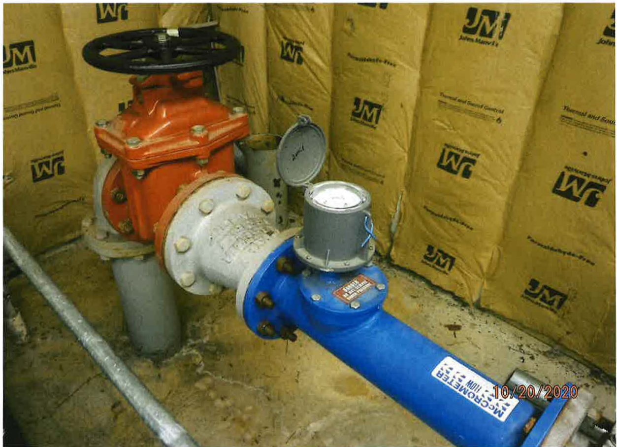
FLOW METER INSTALLED ON WELL 95-95-C-0008
