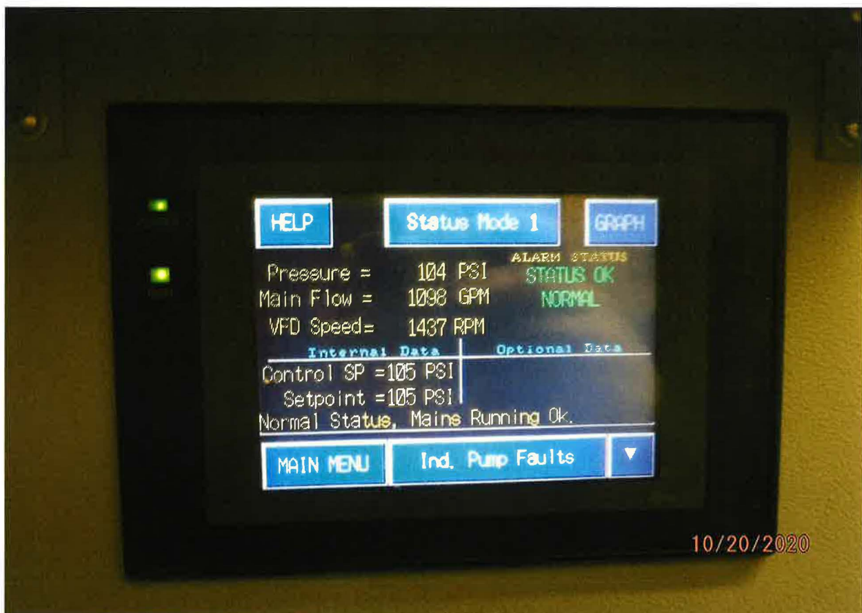
POD - PRE 1960 WELL CONTROL PANEL
