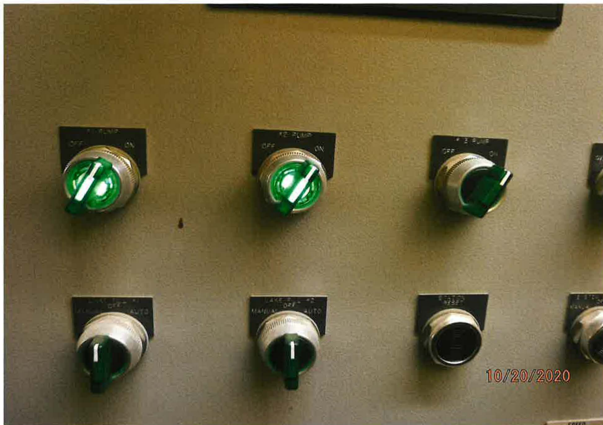
PUMP CONTROL PANEL – 2EA 100 HP PUMPS ACTIVE
