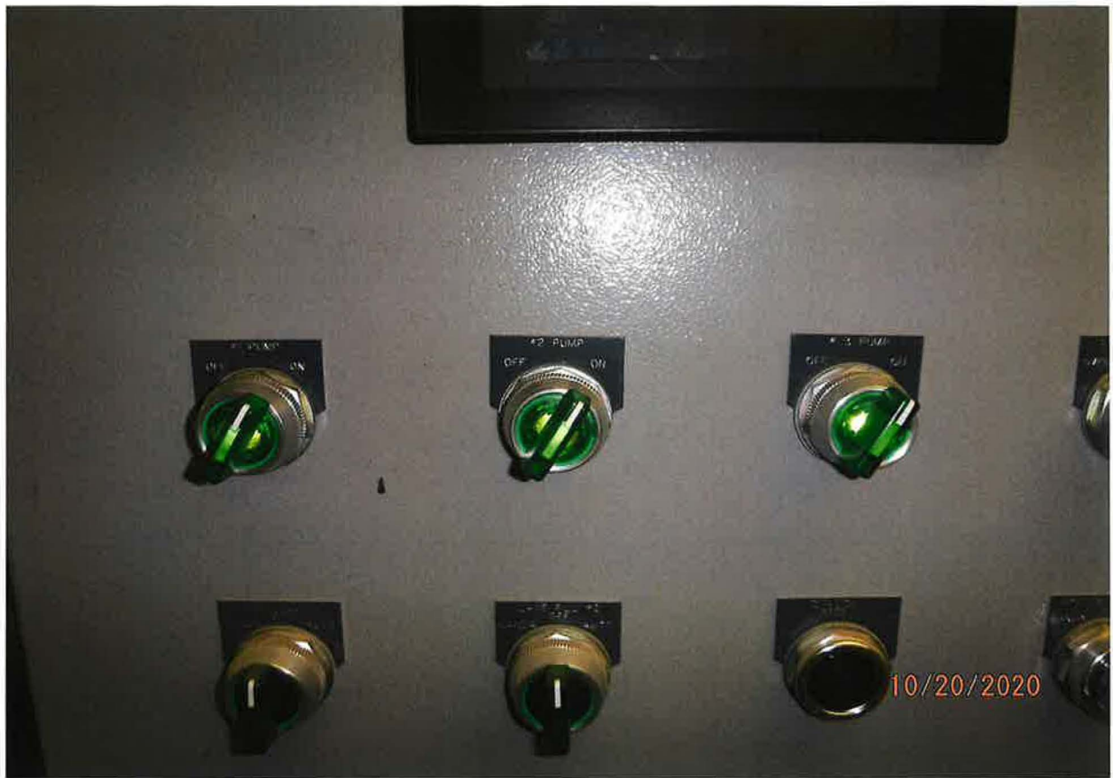
WELL 95-95-C-0008 PUMP 3 ACTIVE
