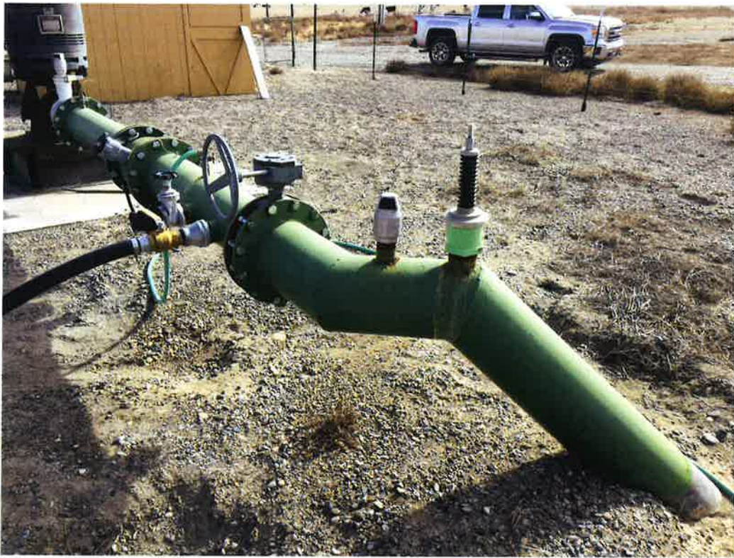
Discharge piping and well pump.
