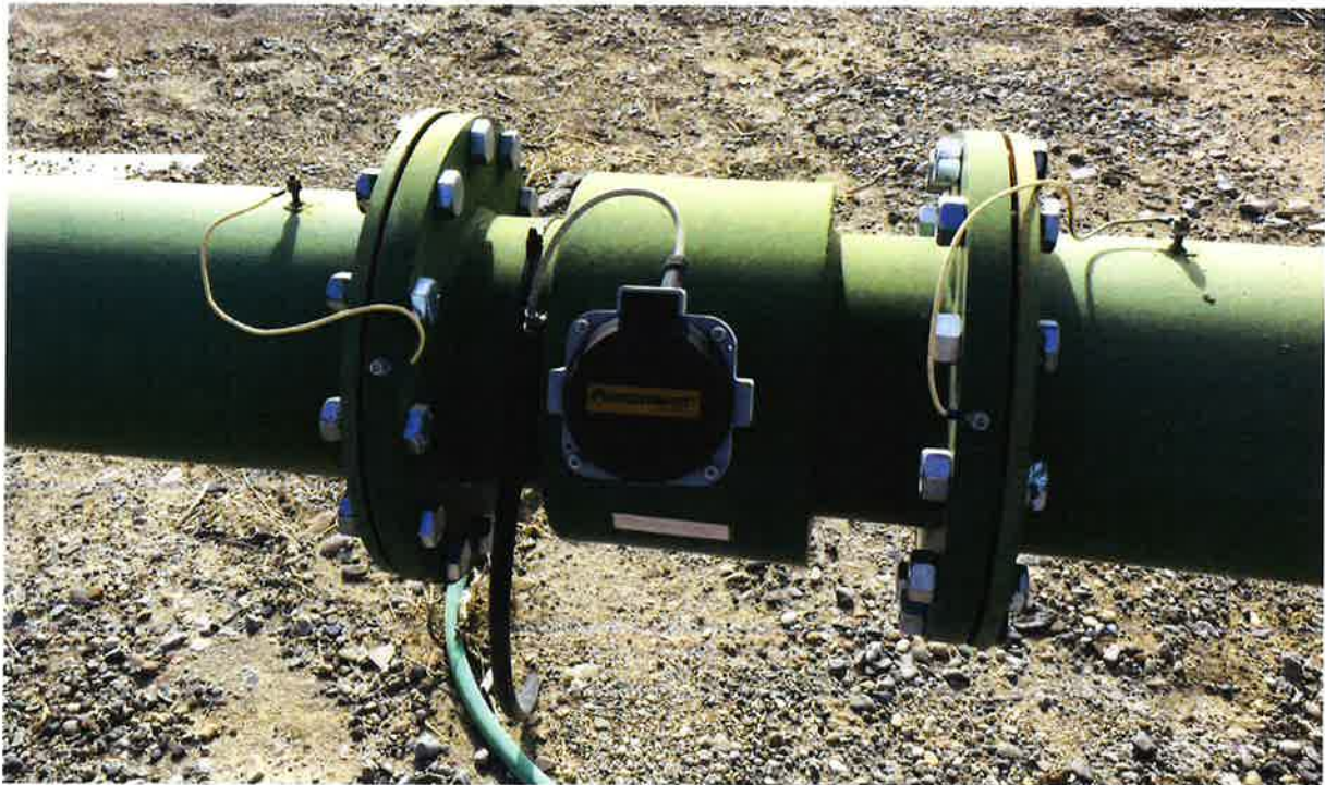
magnetic flow meter on discharge pipe
