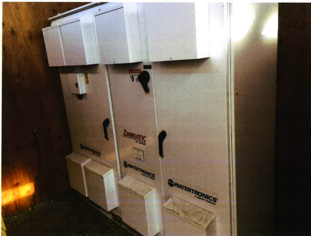
Well pump VFD
