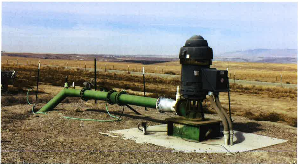
Well with 450-hp vertical turbine pump and discharge piping
