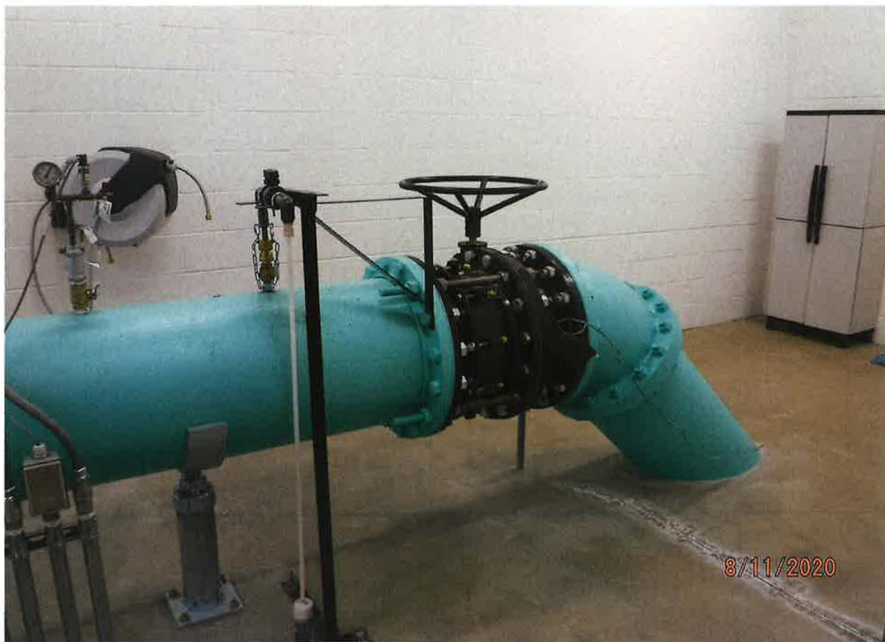
WATER SYSTEM PIPING
