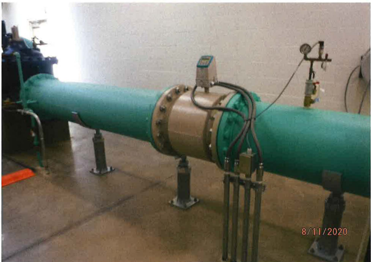
FLOW METER INSTALLED ON WATER SYSTEM
