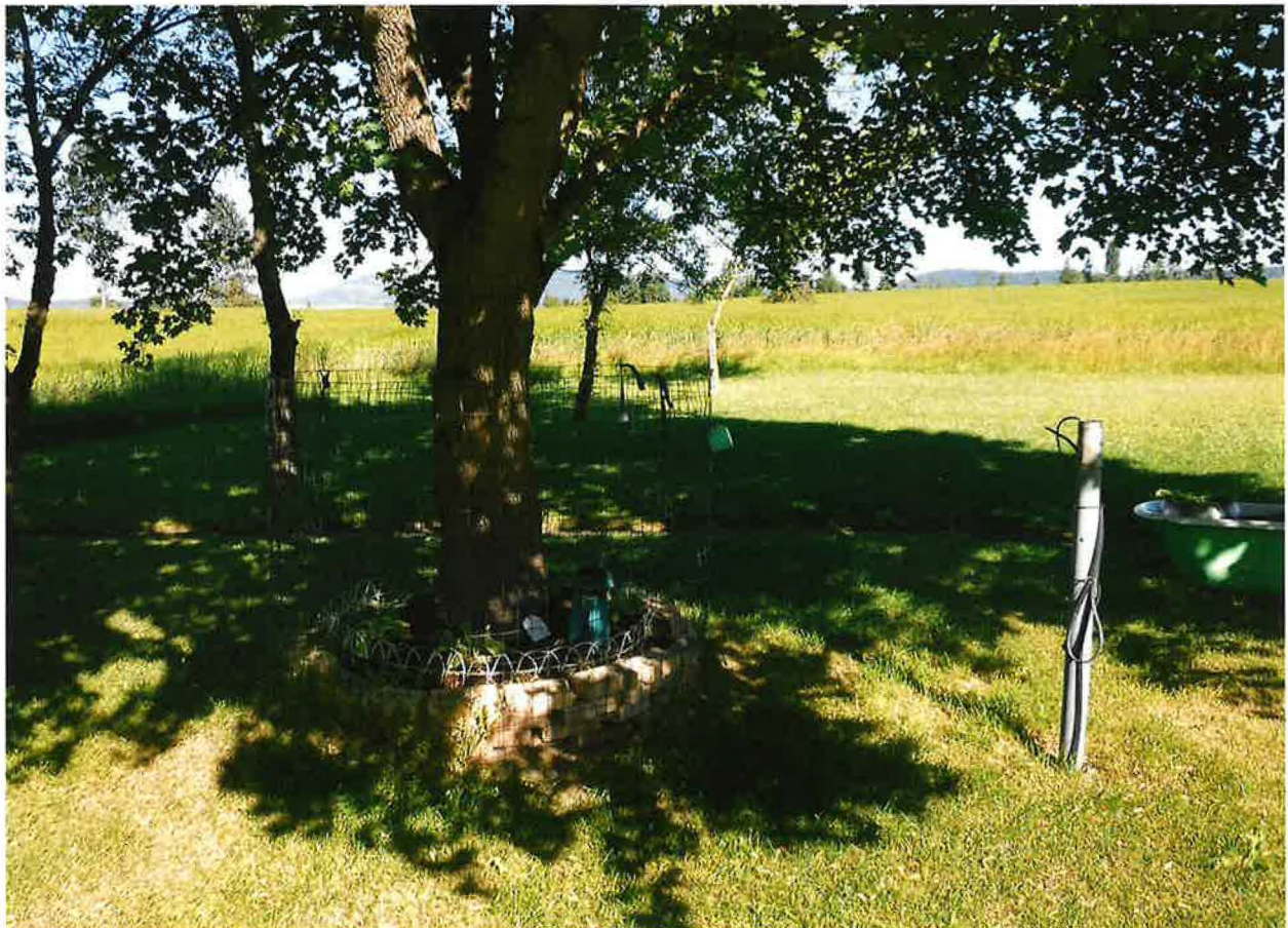
ELECTRICAL STUB FOR GENERATOR TO RUN PUMP FROM POND
