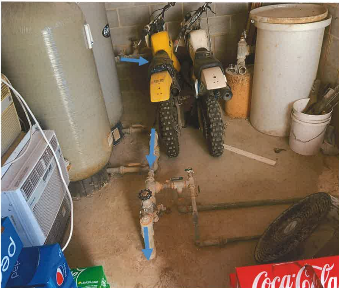
Fig. 4 – View inside of shed. Water comes in from well in background, into the storage tanks, then out via a service line. Abandoned 12" well can be seen in back right corner.
