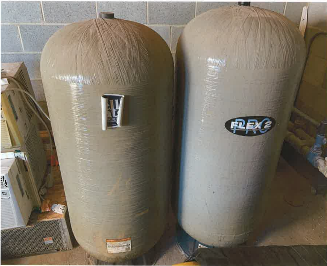
Fig. 5 – Water comes from well to these two holding tanks. According to Down Right Drilling the tanks hold 90 gallons combined.
