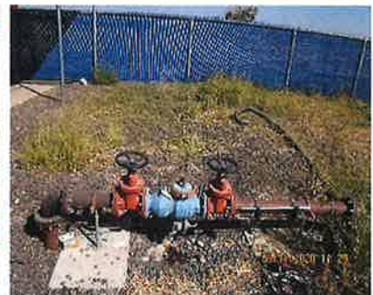
Above ground shutoff and check valves for the well.
