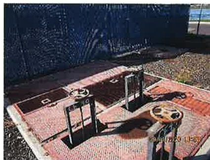
Headgate valves and underground catchment for BCID water.
