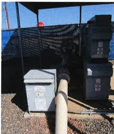
The photo above shows the pumping station. The white pipe diverts BCID water and goes underground where it connects with the 4" pipe from the well.
