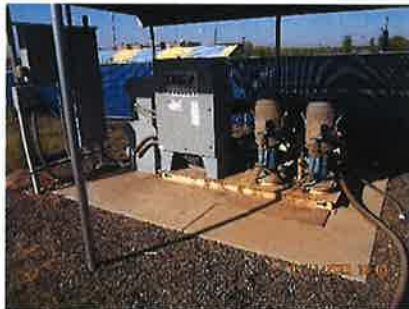
Pumping station. The two pumps in the right of photo are used for BCID water.
