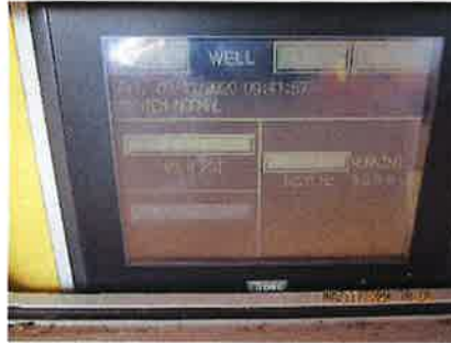
The digital screen at the pumping station. At the site visit, system was running at approximately 70 PSI.
