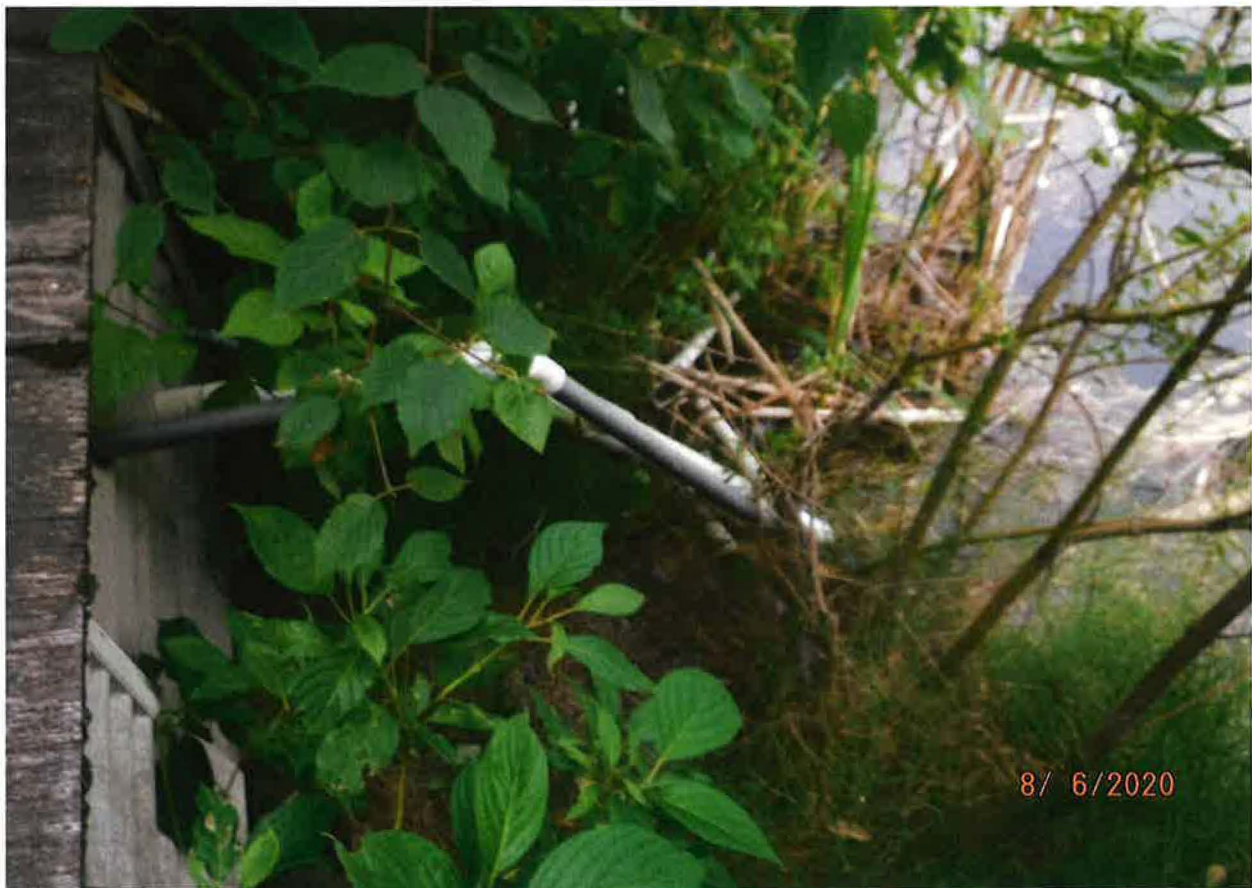
PIPE FROM POND TO PUMP HOUSE FOR IRRIGATION FROM STORAGE USE
