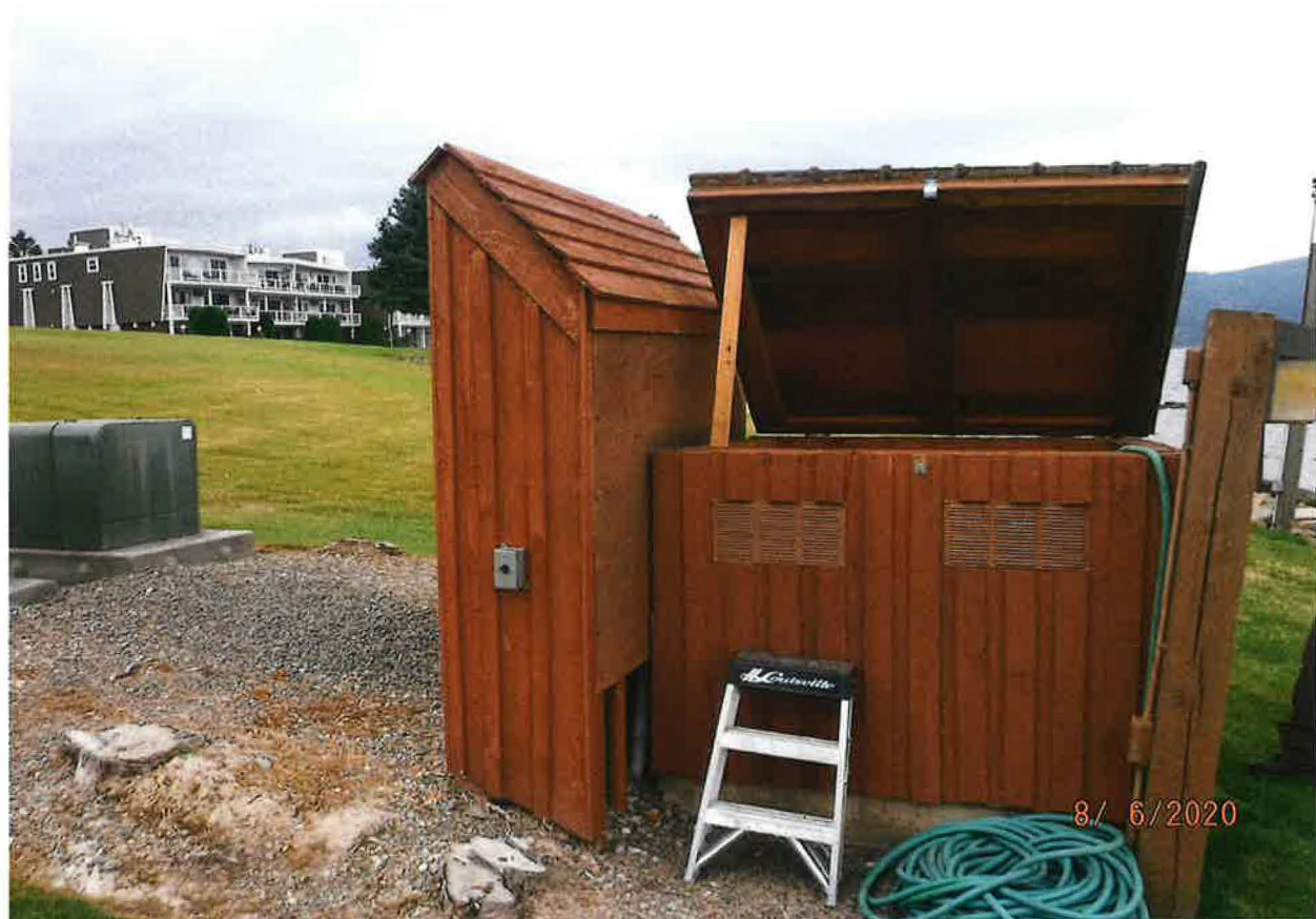
PUMP HOUSE – POD IS AN INTAKE PIPE IN THE PEND OREILLE RIVER
