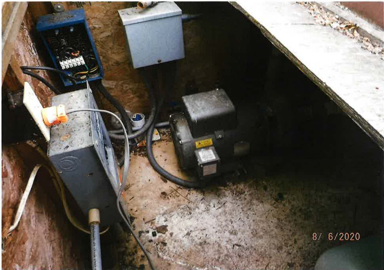
3 HP PUMP USED FOR IRRIGATION FROM STORAGE USE
