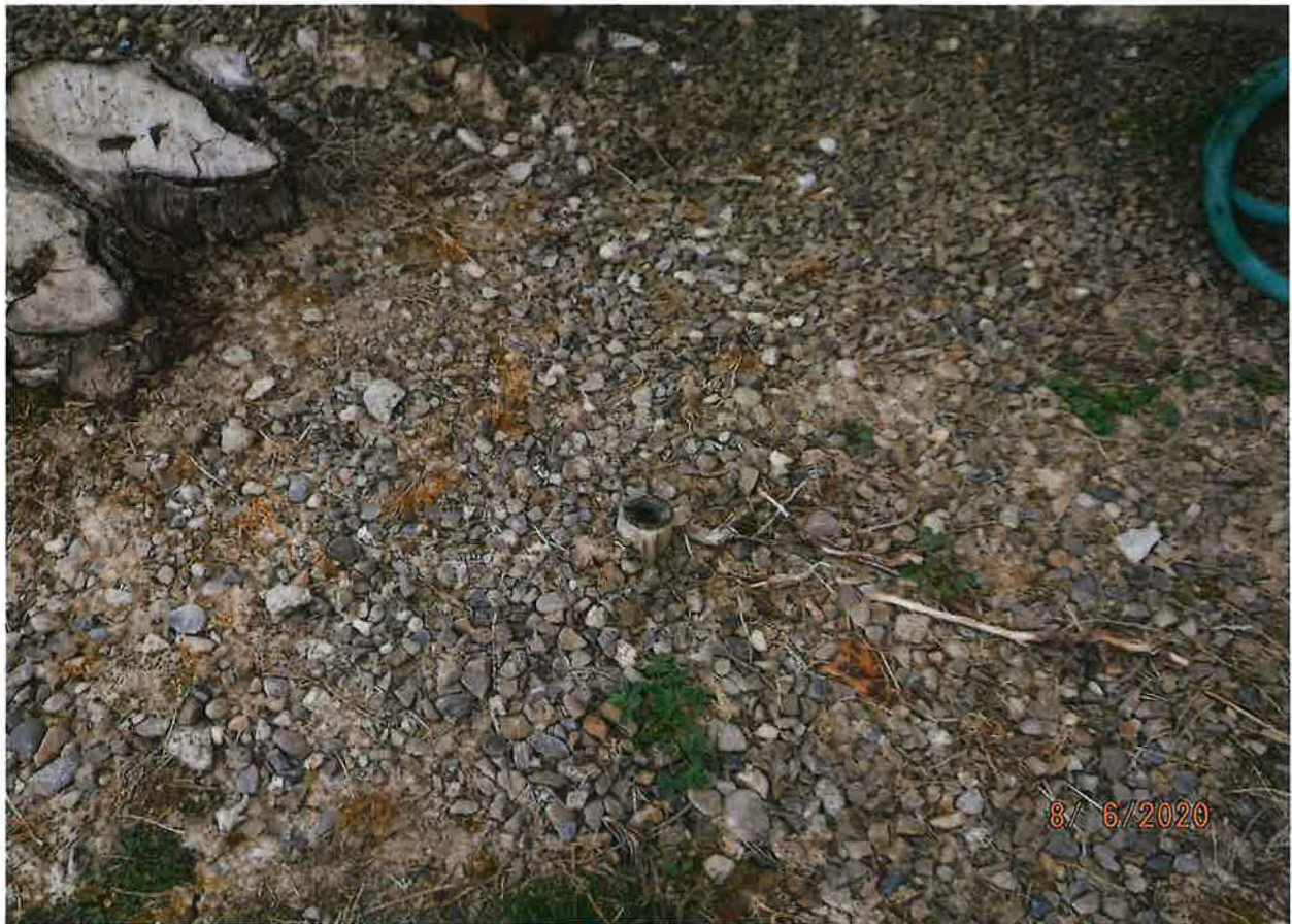
EXAMPLE IRRIGATION RISER FOR PRESSURIZED SPRINKLERS
