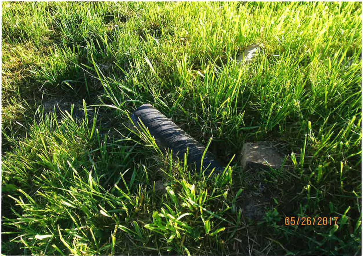
OVERFLOW DISCHARGE PIPE FROM POND
