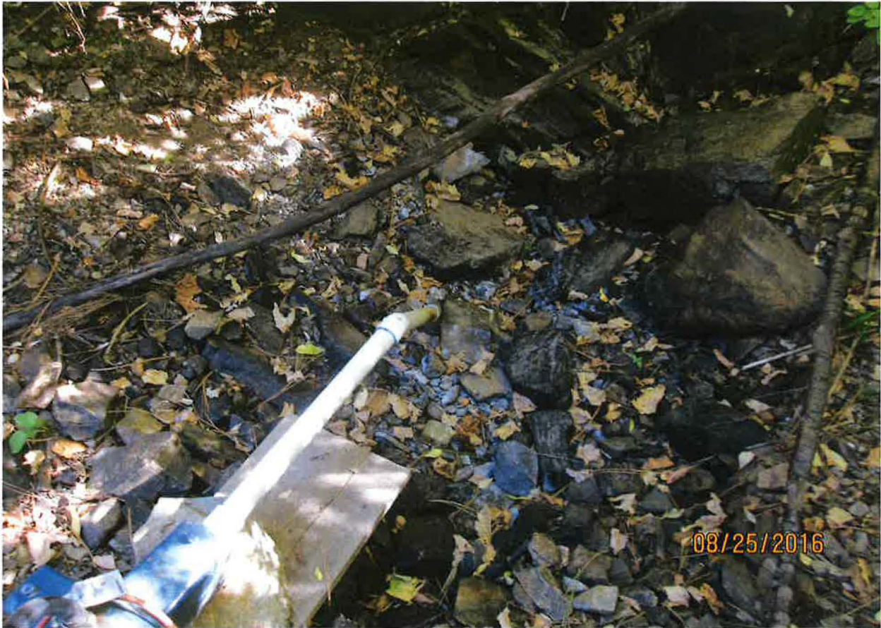
POD – PUMP WITH INTAKE PIPE IN UNNAMED STREAM
