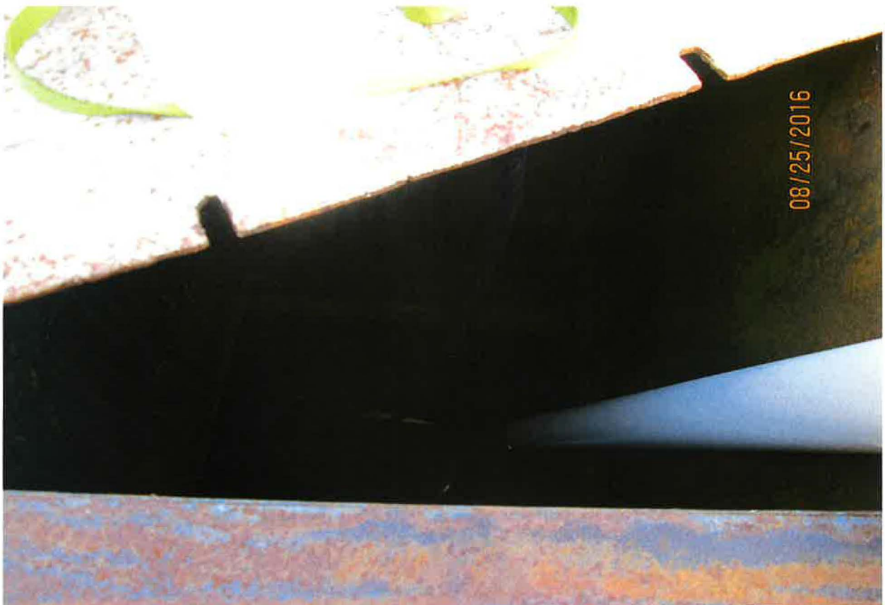
SUB-SURFACE STORAGE TANK, LESS THAN 500 GALLON CAPACITY
