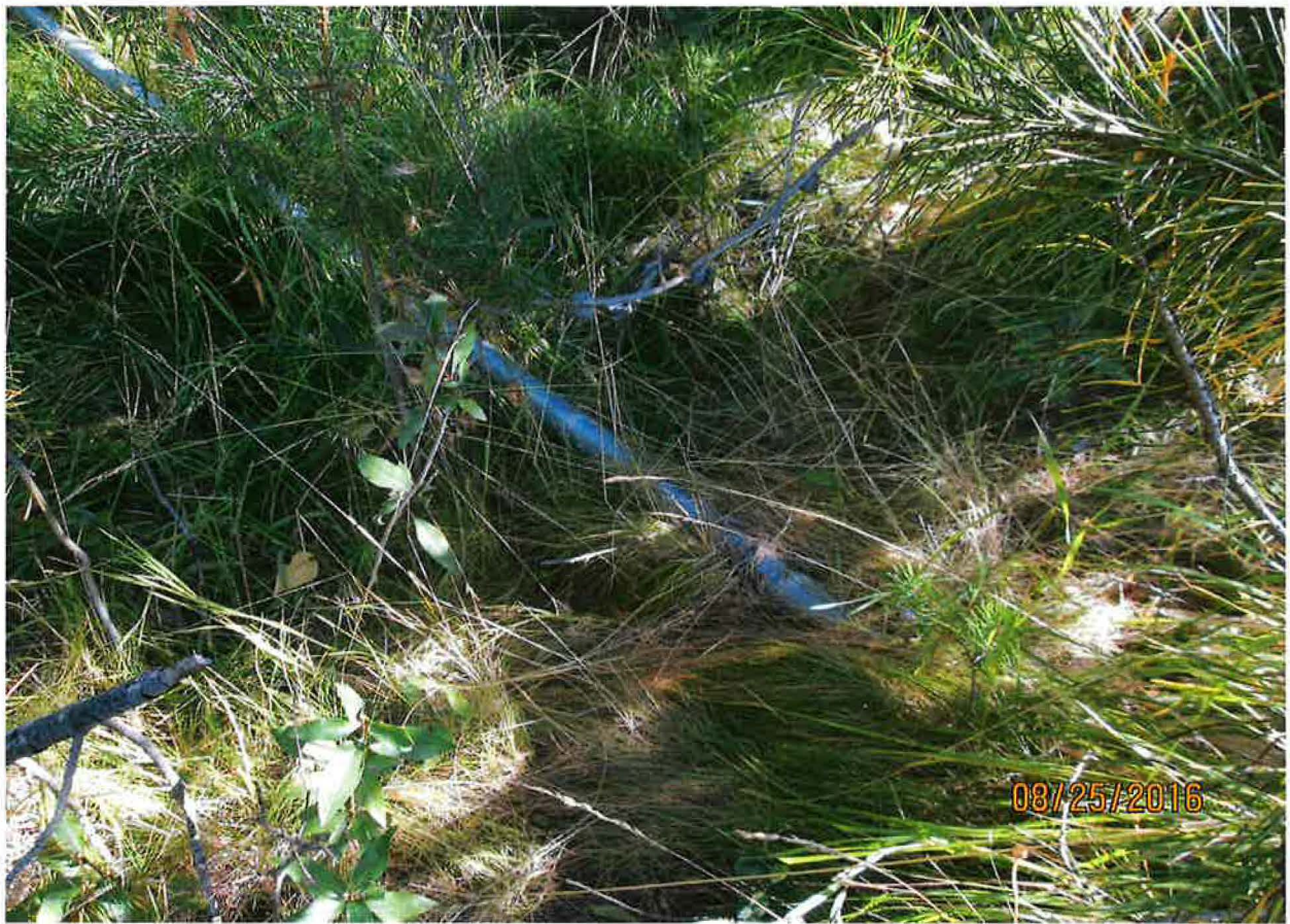
WATER SYSTEM PIPE ROUTED BENEATH ROAD TO SMALL STORAGE TANK
