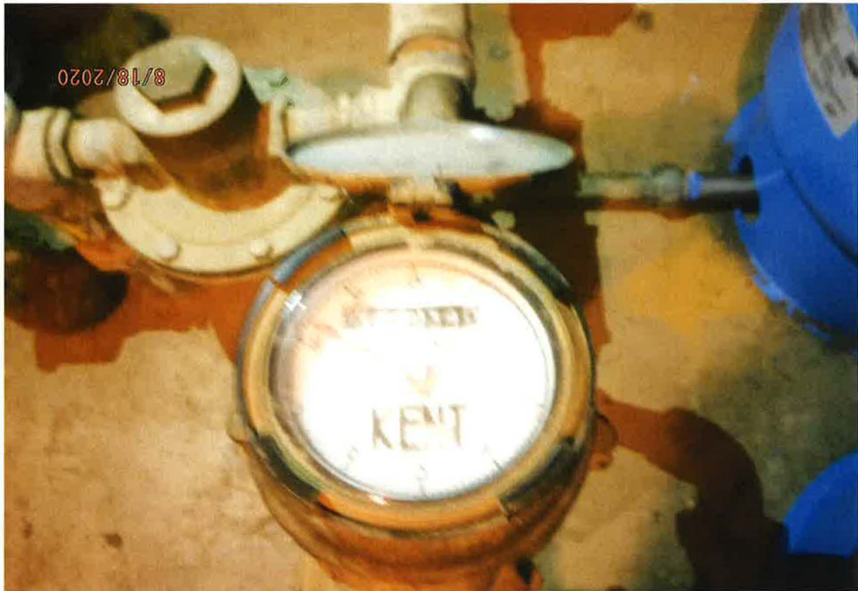
FLOWMETER INSTALLED ON SYSTEM
