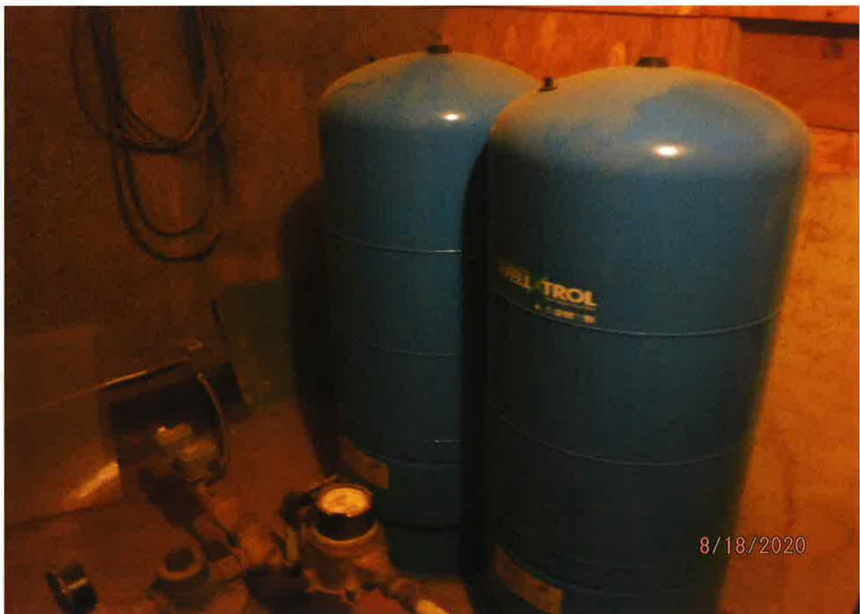
2EA PRESSURE TANKS DIRECT LINE FROM WELL
