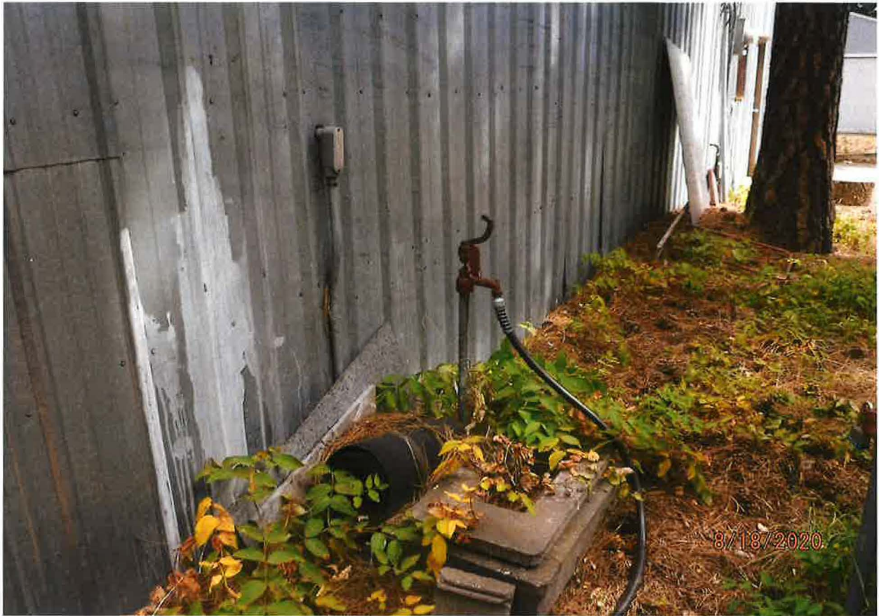
FIRE PROTECTION POU – FROST FREE HYDRANTS POSITIONED THROUGHOUT COMMERCIAL PARK
