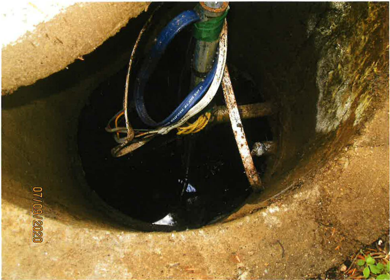
POD - CONCRETE CISTERN COLLECTING GROUNDWATER
