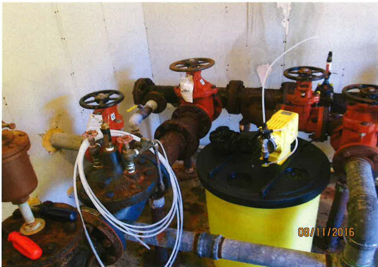
WATER CONVEYANCE SYSTEM PIPES
