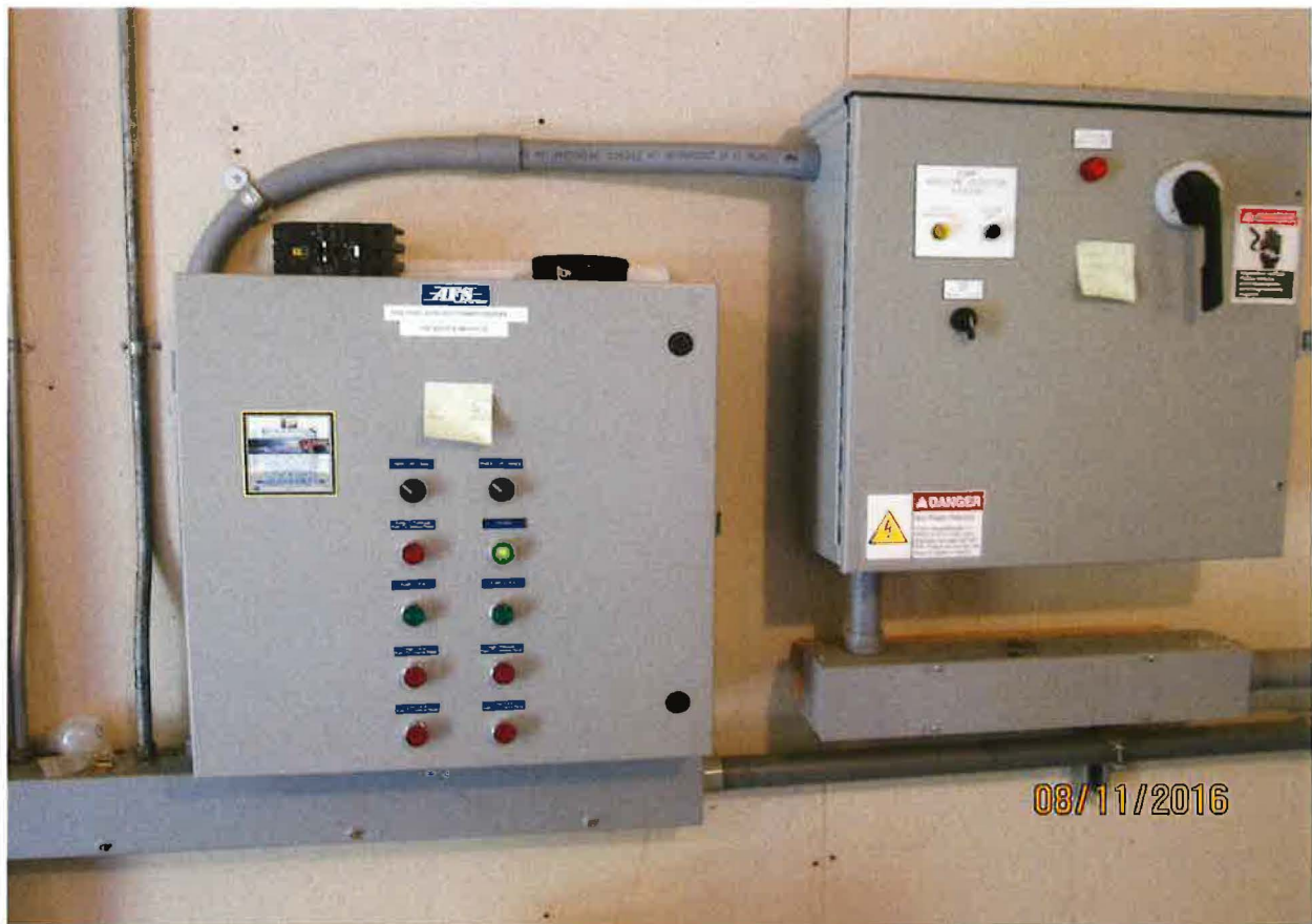
SYSTEM CONTROL PANEL – 40 HP PUMP INSTALLED WELL D0013791
