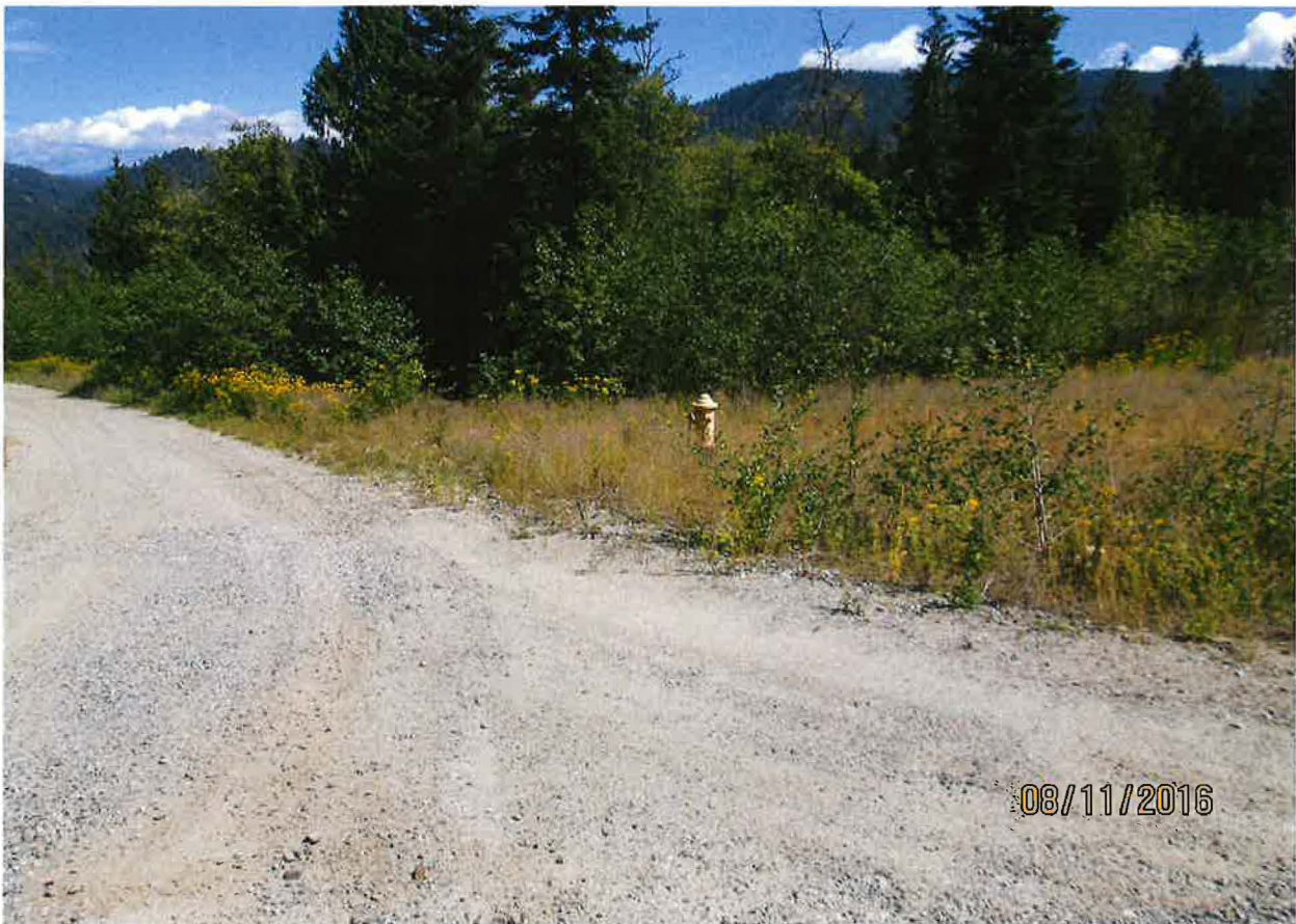
EXAMPLE - FIRE SYSTEM INSTALLED FIRE HYDRANT IN MUNICIPAL POU
