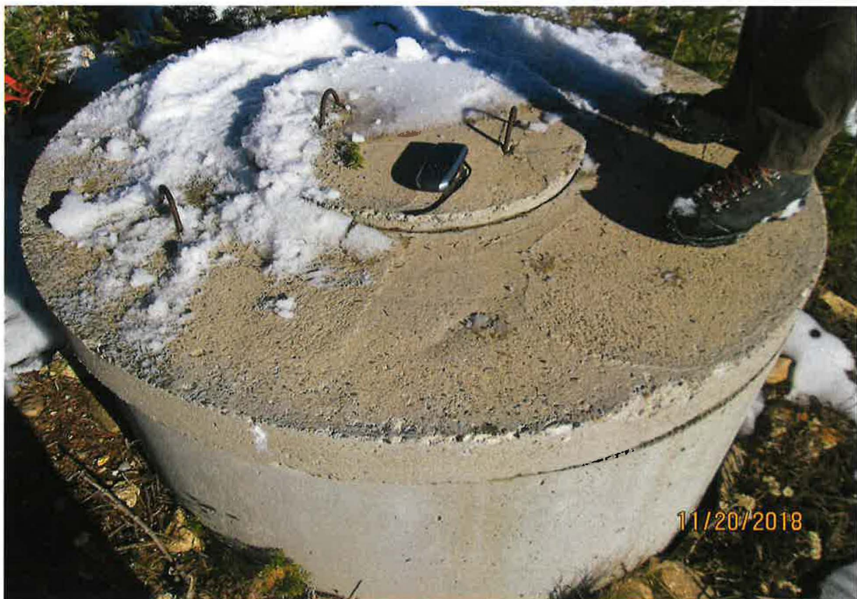
POD – WELL A0020030 (ENCASED WITH CONCRETE FOR PROTECTION)
