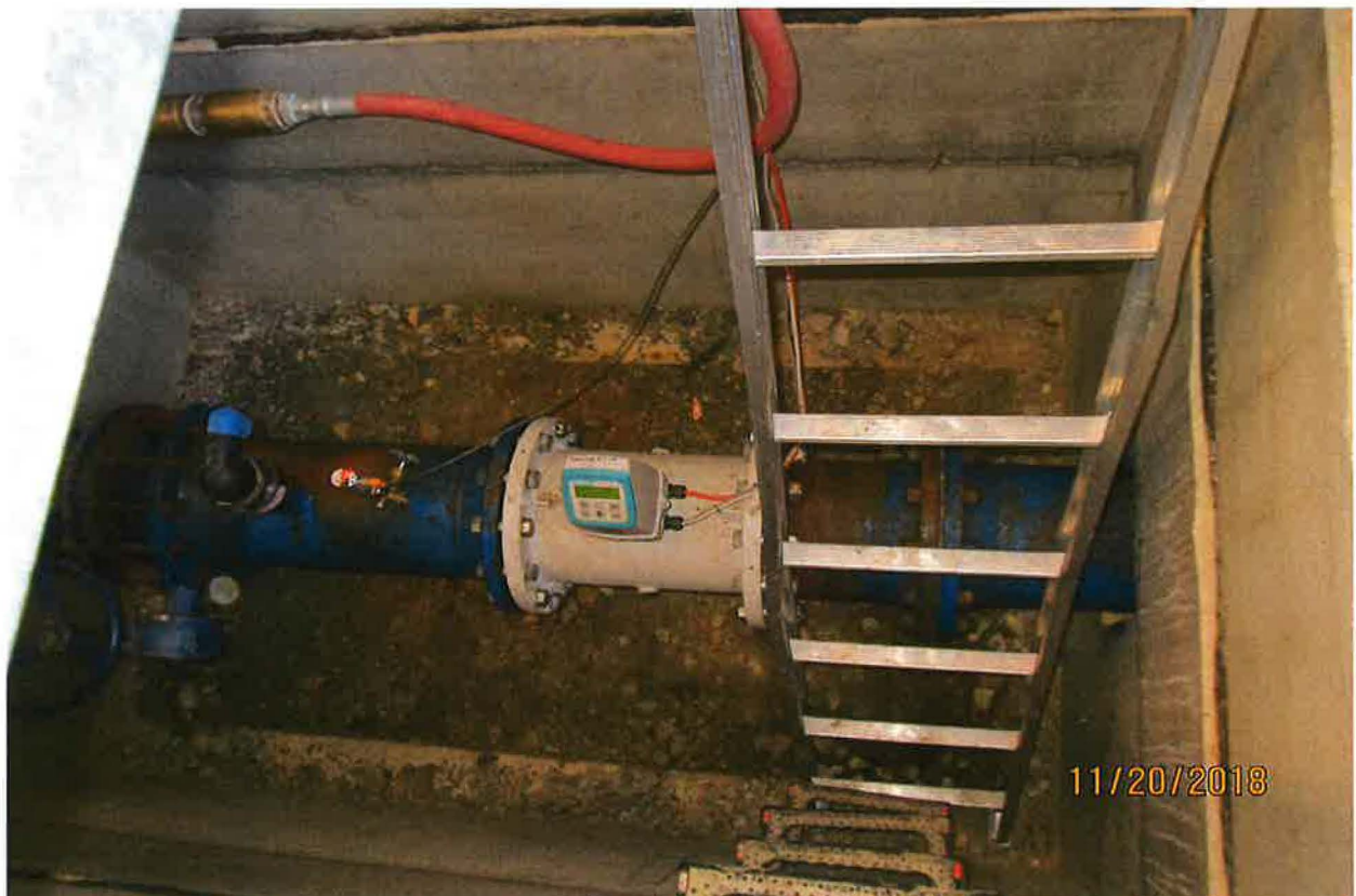
FLOWMETER INSTALLED ON MAINLINE
