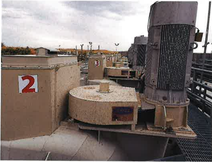
View of Turbines looking Northeast
