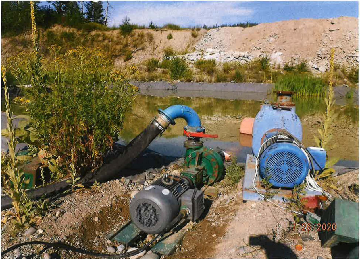
RECIRCULATION PUMP BACK TO INDUSTRIAL OPERATIONS
