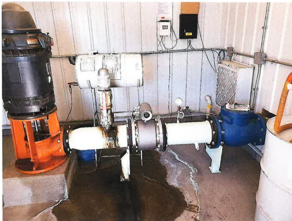
Figure 4: Photo inside pump house from IDWR 2020 visit
