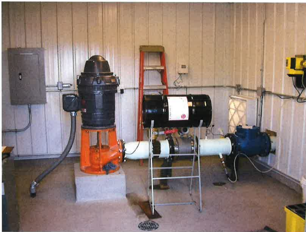
Figure 2: Pump and meter assembly in well house (photo provided by Karen Henderson)
