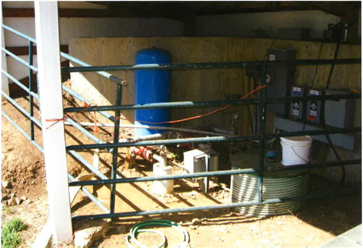
PUMP SYSTEM FOR IRRIGATING FROM 24HR IMPOUNDMENT POND
