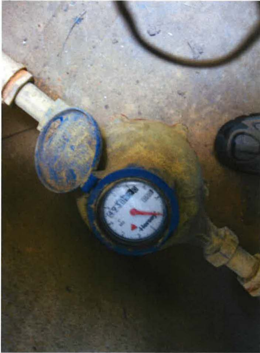
FLOW METER INSTALLED ON IRRIGATION SYSTEM
