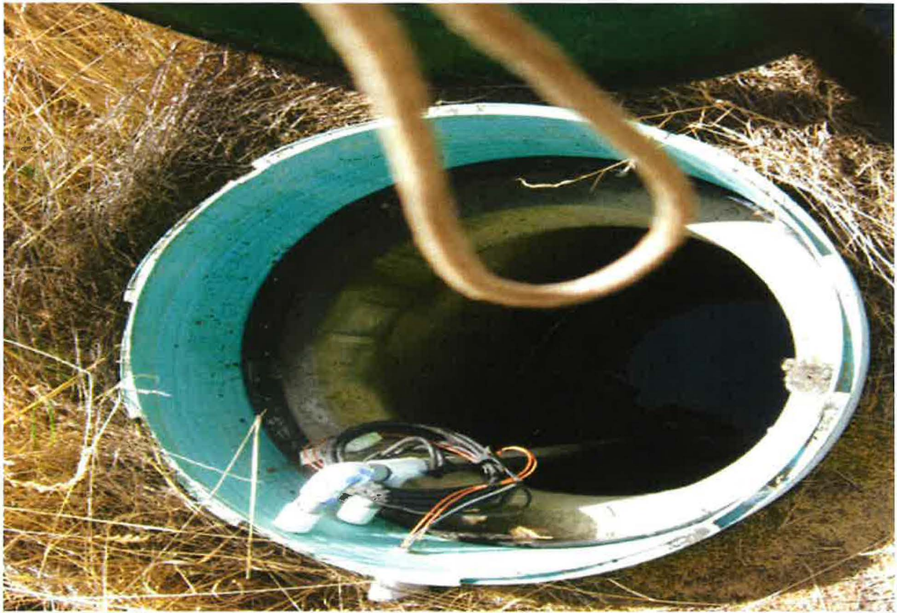
WET WELL AT FIRST STAGE PUMP HOUSE – INCLUDES BOOSTER PUMP TO ROUTE WATER UP-HILL TO POU
