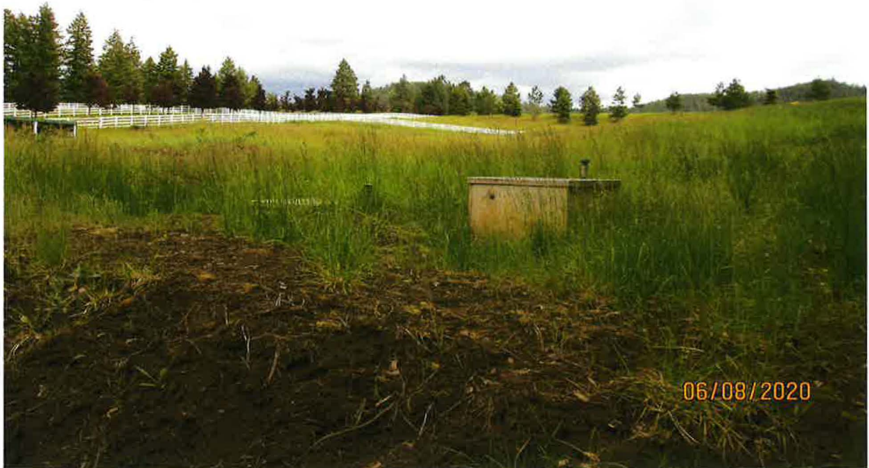
2 EACH 3,000 GALLON VAULTED STORAGE TANKS
