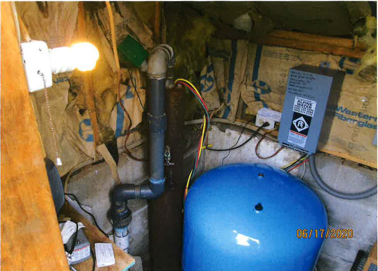
PUMP HOUSE CONTAINING PRESSURE TANK FOR WATER SYSTEM
