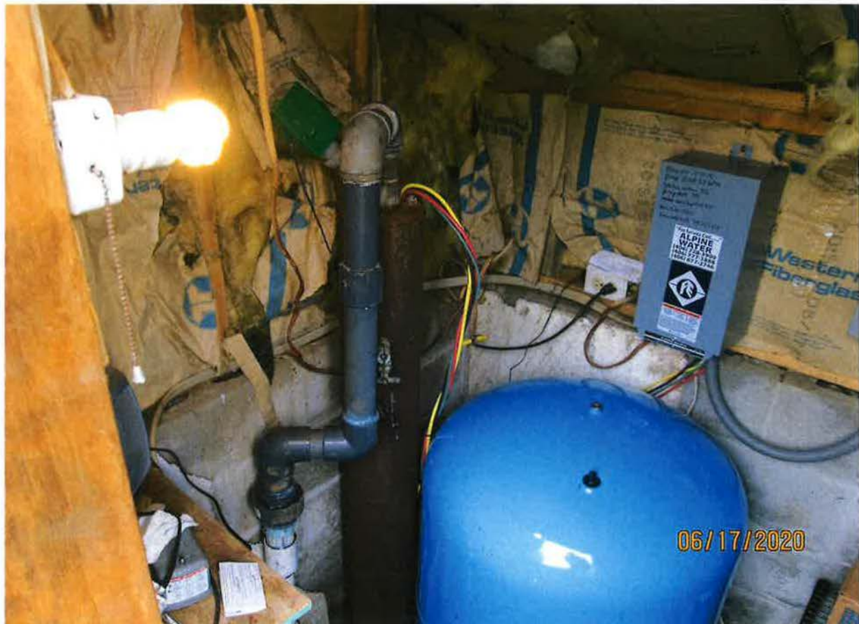
POD - WELL 94-93-N-23-000
