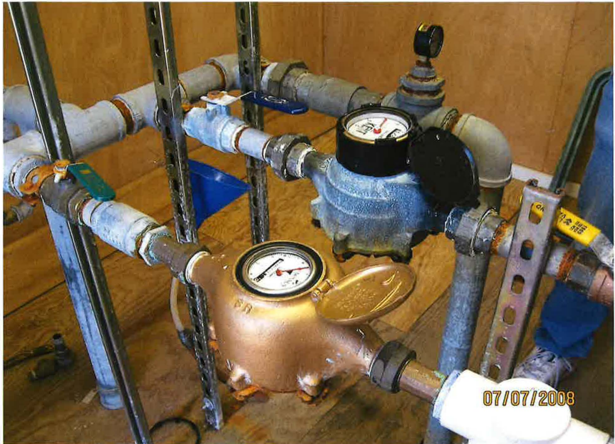
FLOW METERS INSTALLED ON EACH WELL PRIOR TO DISTRIBUTION TO STORAGE TANK
