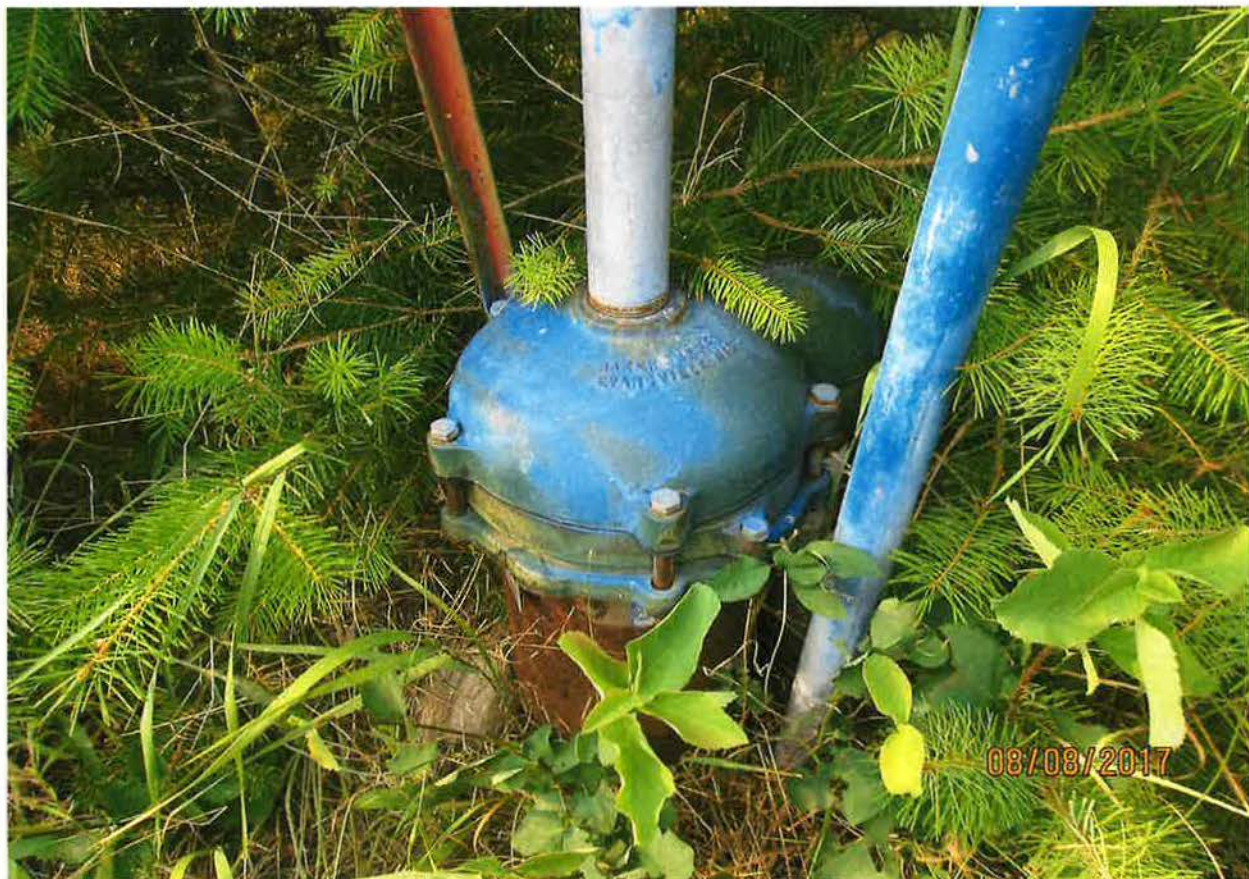
POD - WELL D0003345
