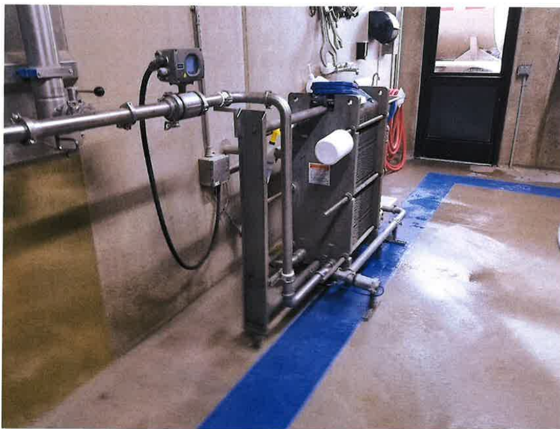
Looking at plate cooler (rarely used per Applicant).
