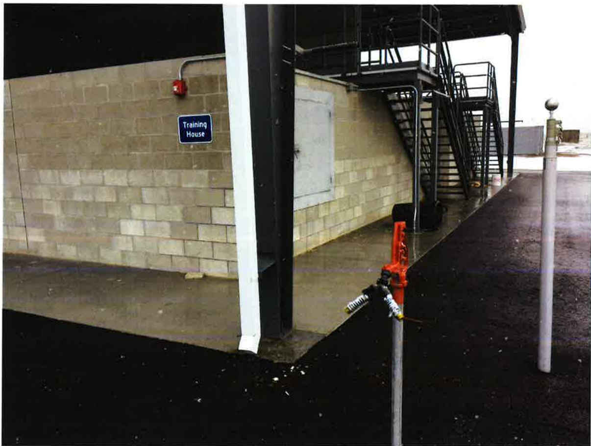
Yard hydrant at training house
