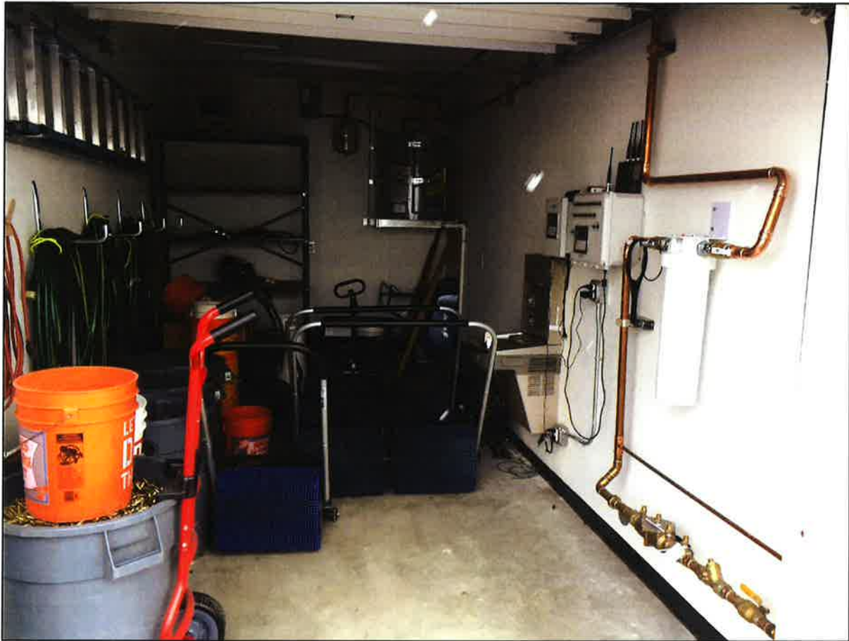
Mechanical room at satellite restroom building.
