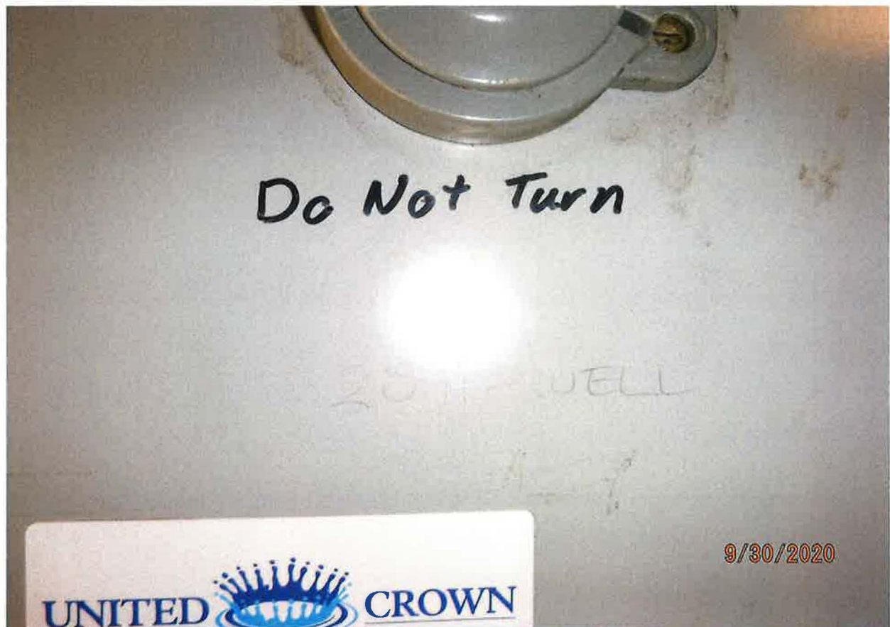
25 HP PUMP IN WELL 95-89-N-44
