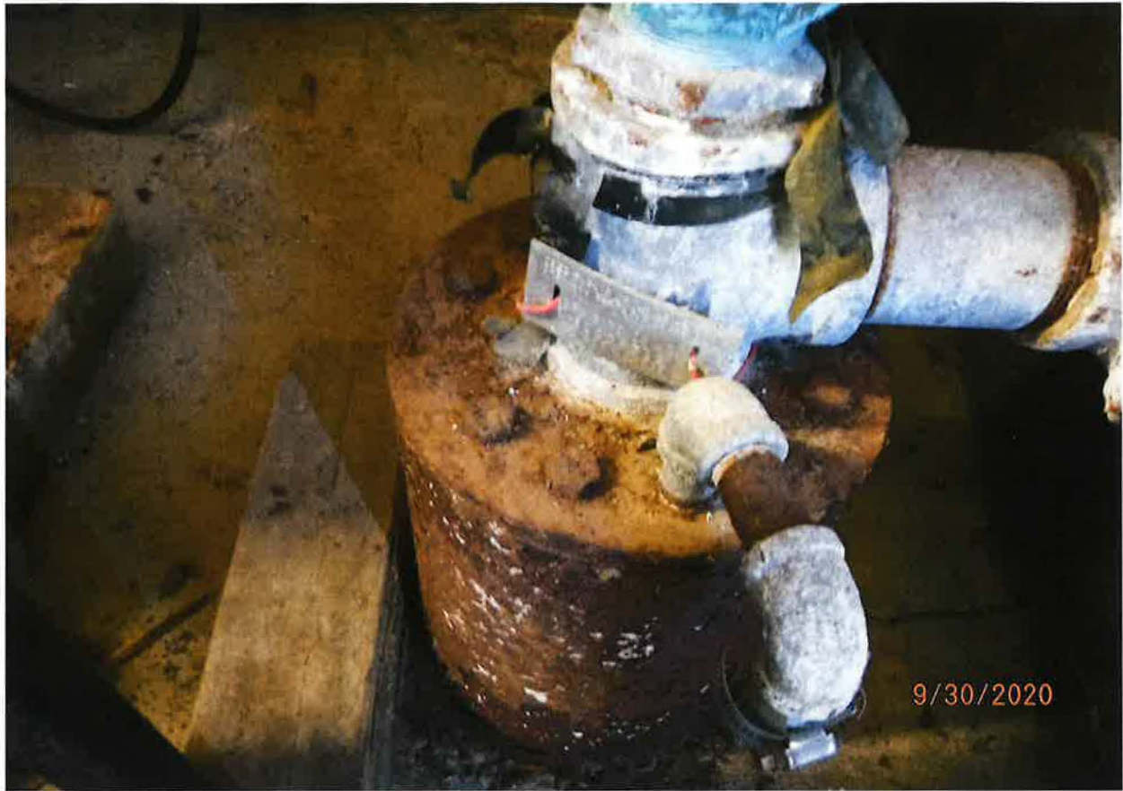
POD – WELL IN PUMP HOUSE (E0005319)
