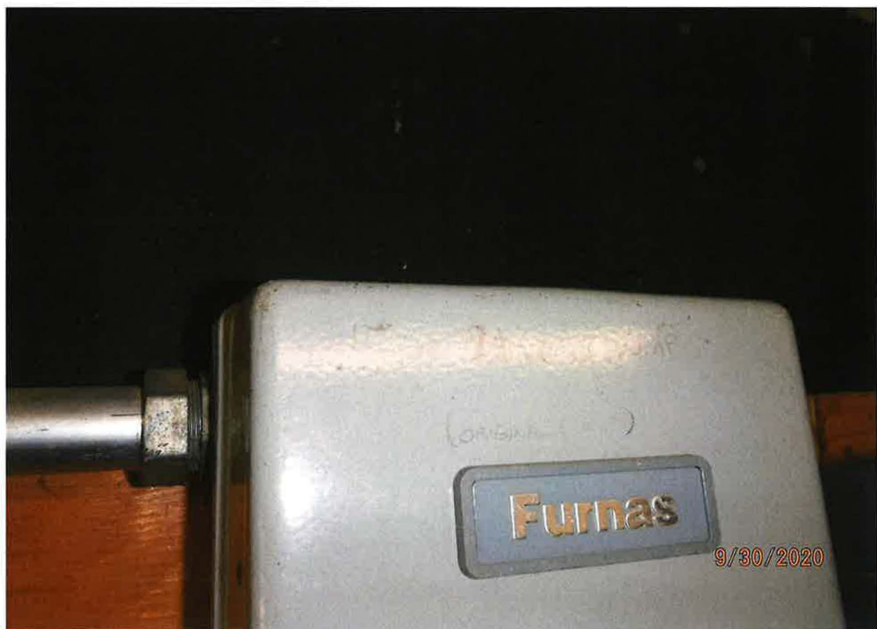
15 HP PUMP IN WELL LOCATED IN PUMPHOUSE – NO TAG INFORMATION
