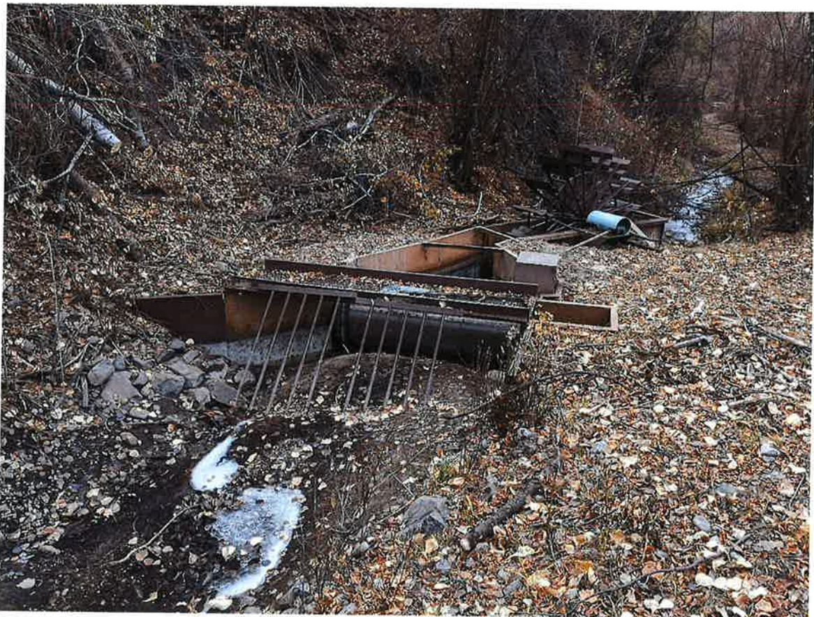
Photo 2: Fish screen structure
