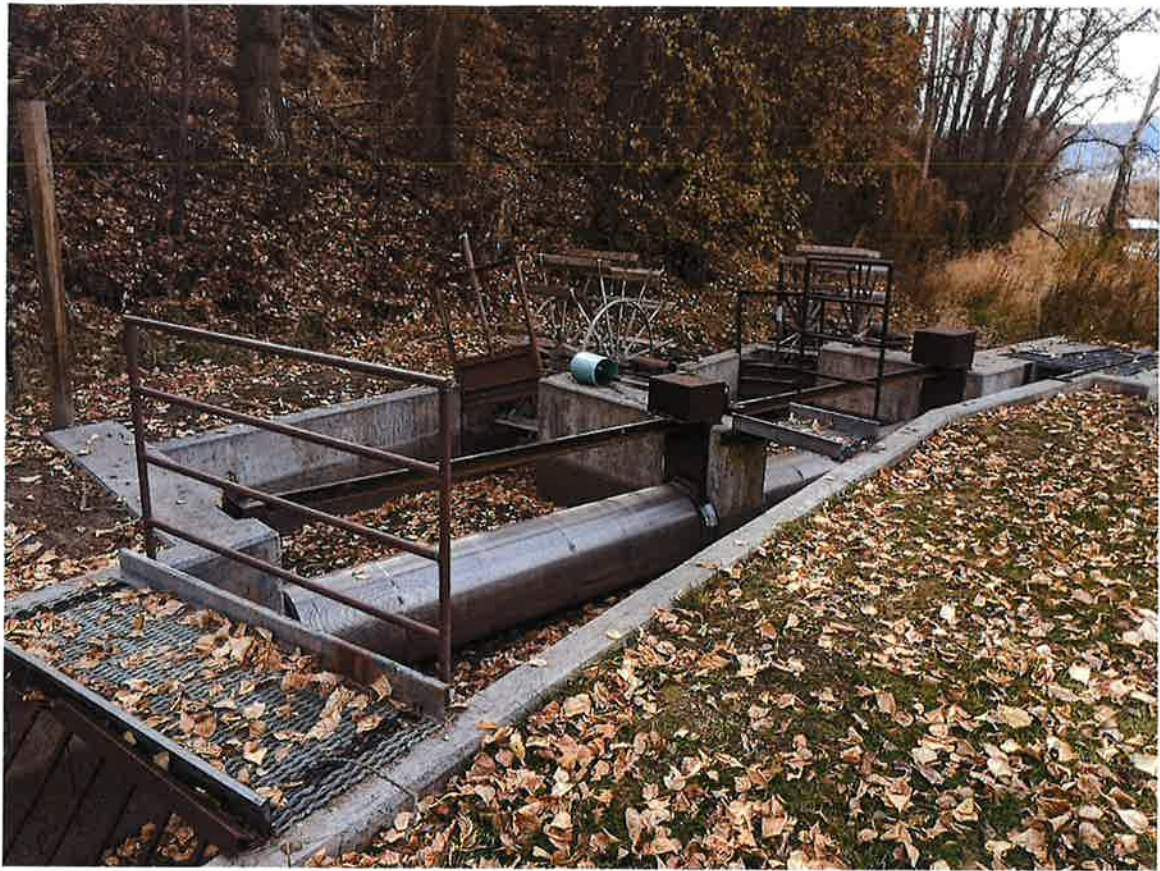
Photo 3: Fish screen structure
