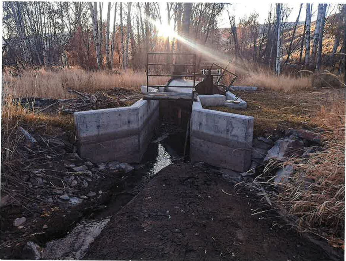
Photo 2: Fish screen/bypass approach
