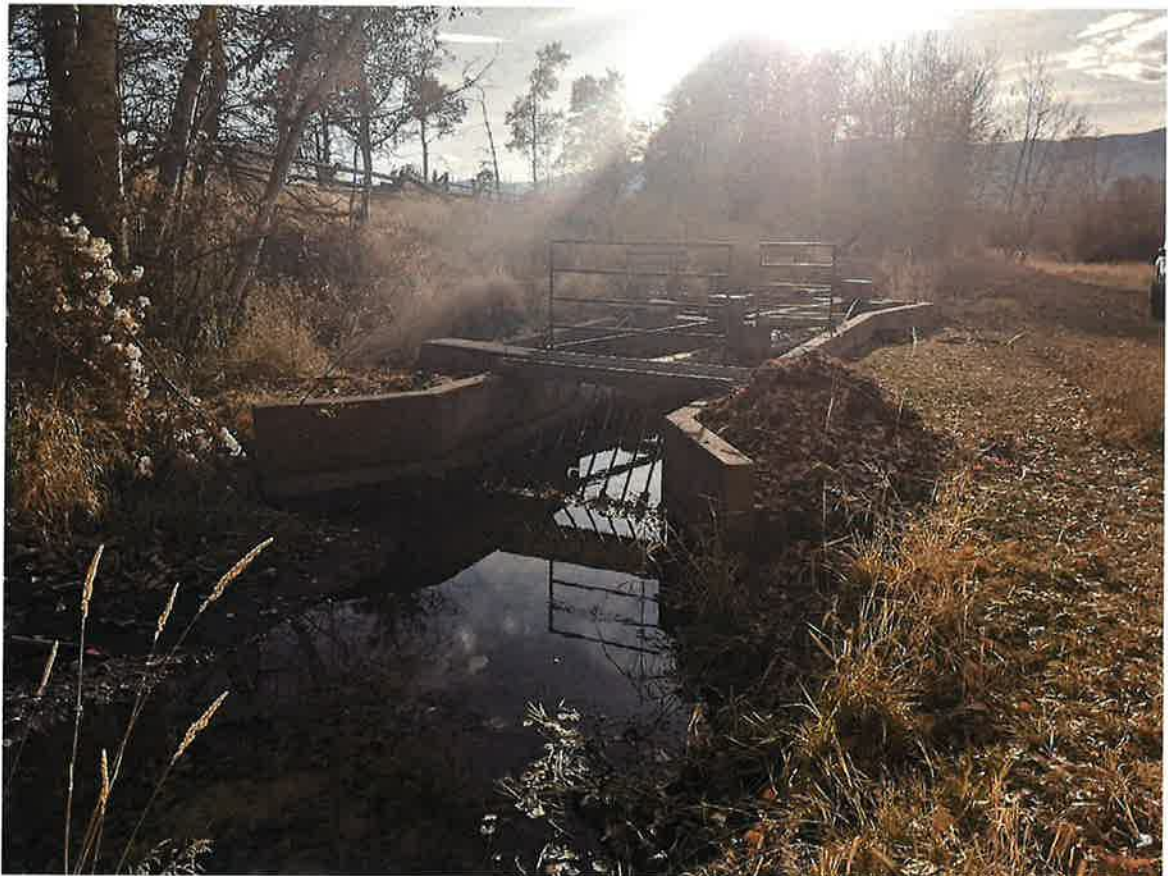
Photo 2: Fish screen/bypass approach
