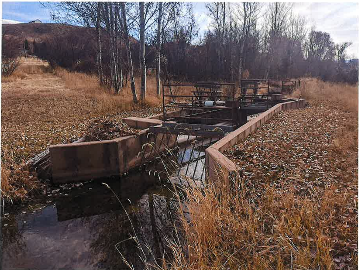
Photo 2: Fish screen/bypass approach
