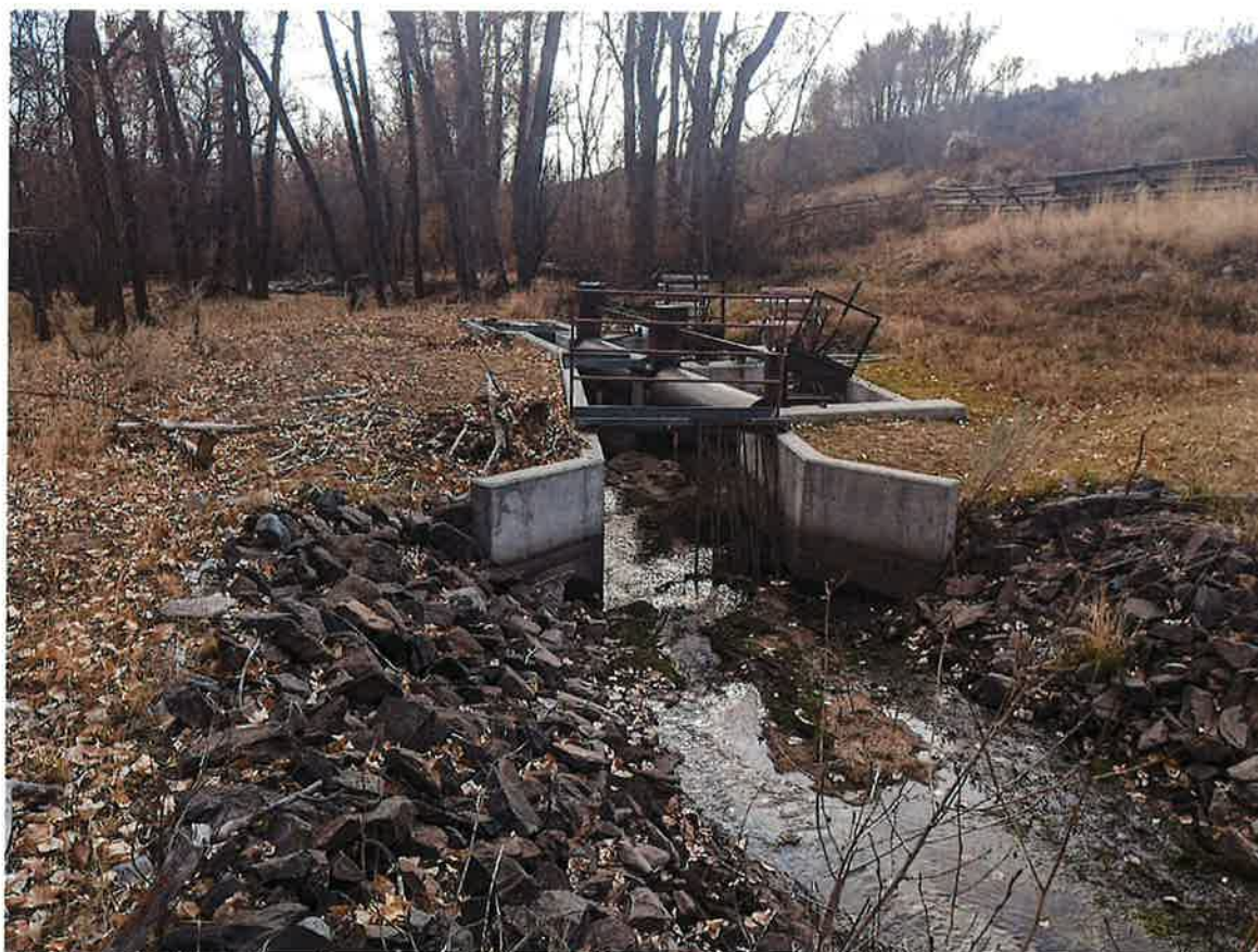
Photo 2: Fish screen/bypass approach
