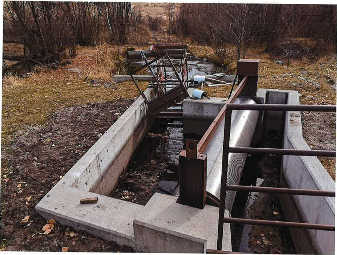
Photo 3: Fish screen structure
