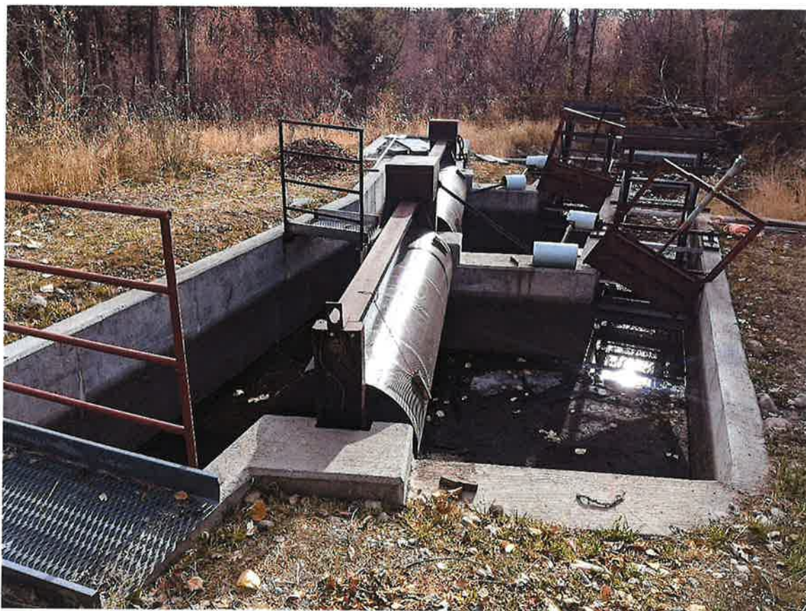
Photo 3: Fish screen structure
