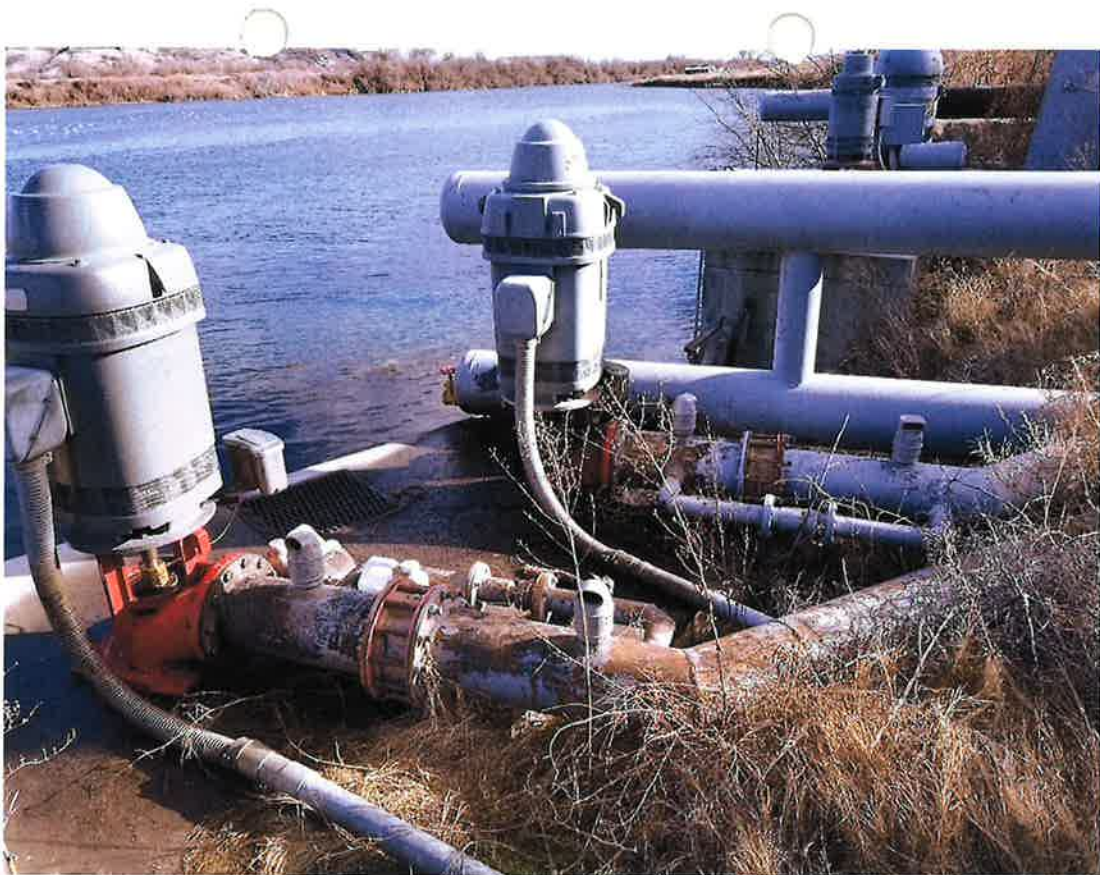
Looking at Snake River pump station 1,050 HP total (4 pumps - 2 pumps per 16 inch OD penstock)
