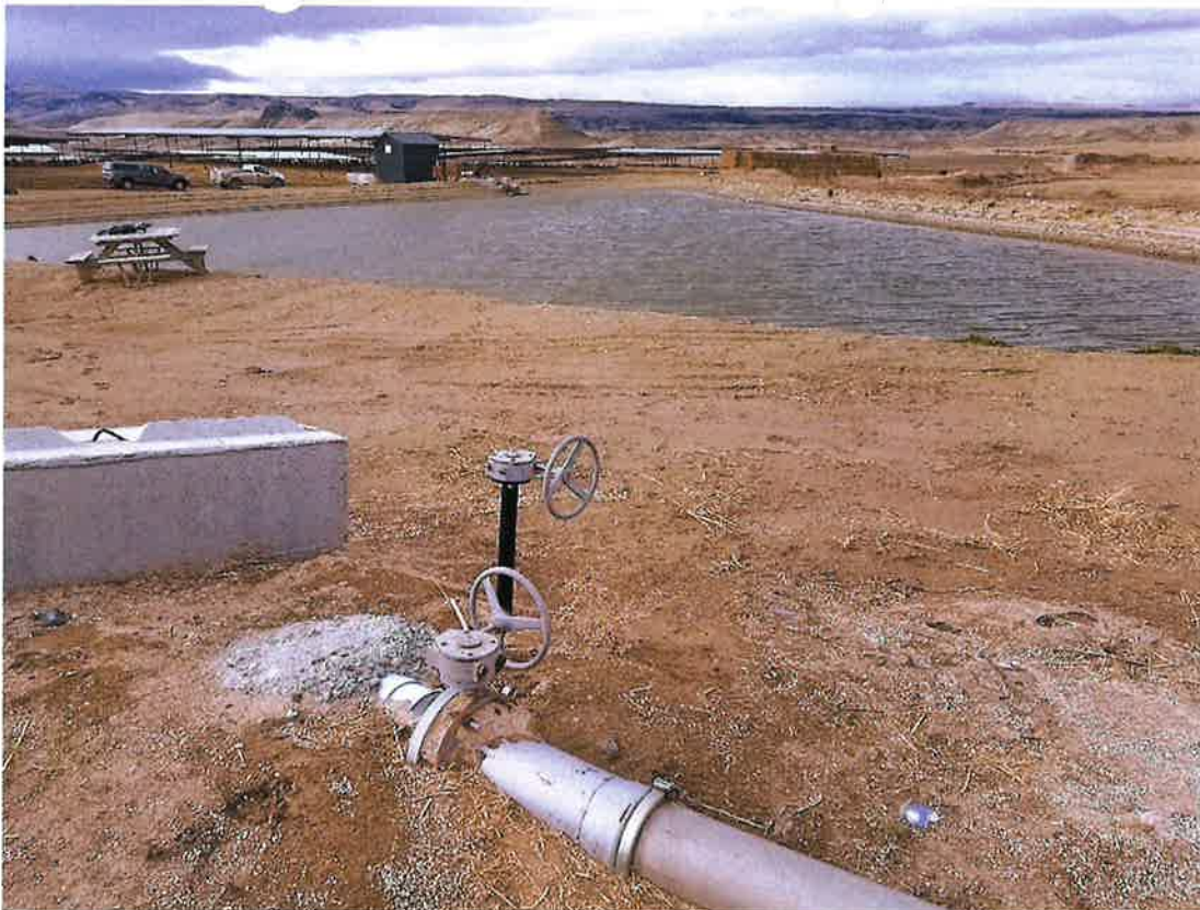
Looking at valves to fill holding pond with Snake River water and well water if needed (green treatment shed can be seen directly across pond).
