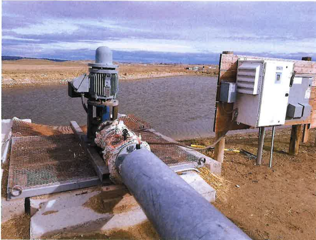
Looking at holding pond that is filled with Snake River water. Water is pumped out of holding pond into a water treatment facility where it is chemically treated and used within the dairy.
