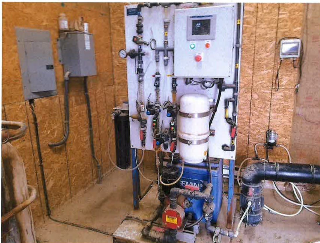
Looking at chemical treatment facility for Snake River water being pumped from adjacent holding pond.
