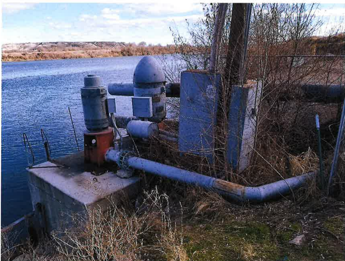
Looking at Snake River pump station 1,050 HP total (4 pumps - 2 pumps per 16 inch OD penstock)
