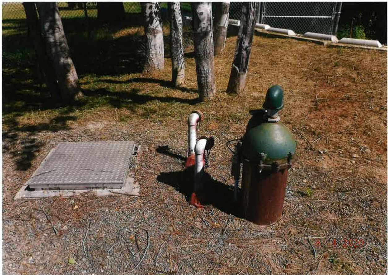
POD - WELL No. 1 - NO TAG, 20 HP PUMP
