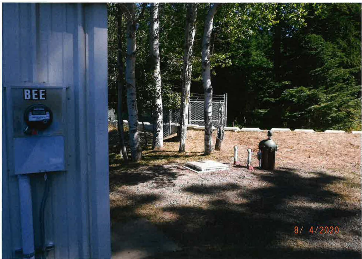
PUMP STATION CO-LOCATED WITH WELL No. 1
