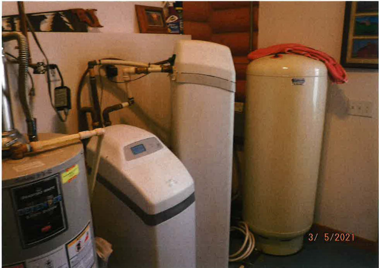
WATER SYSTEM PRESSURE TANK
