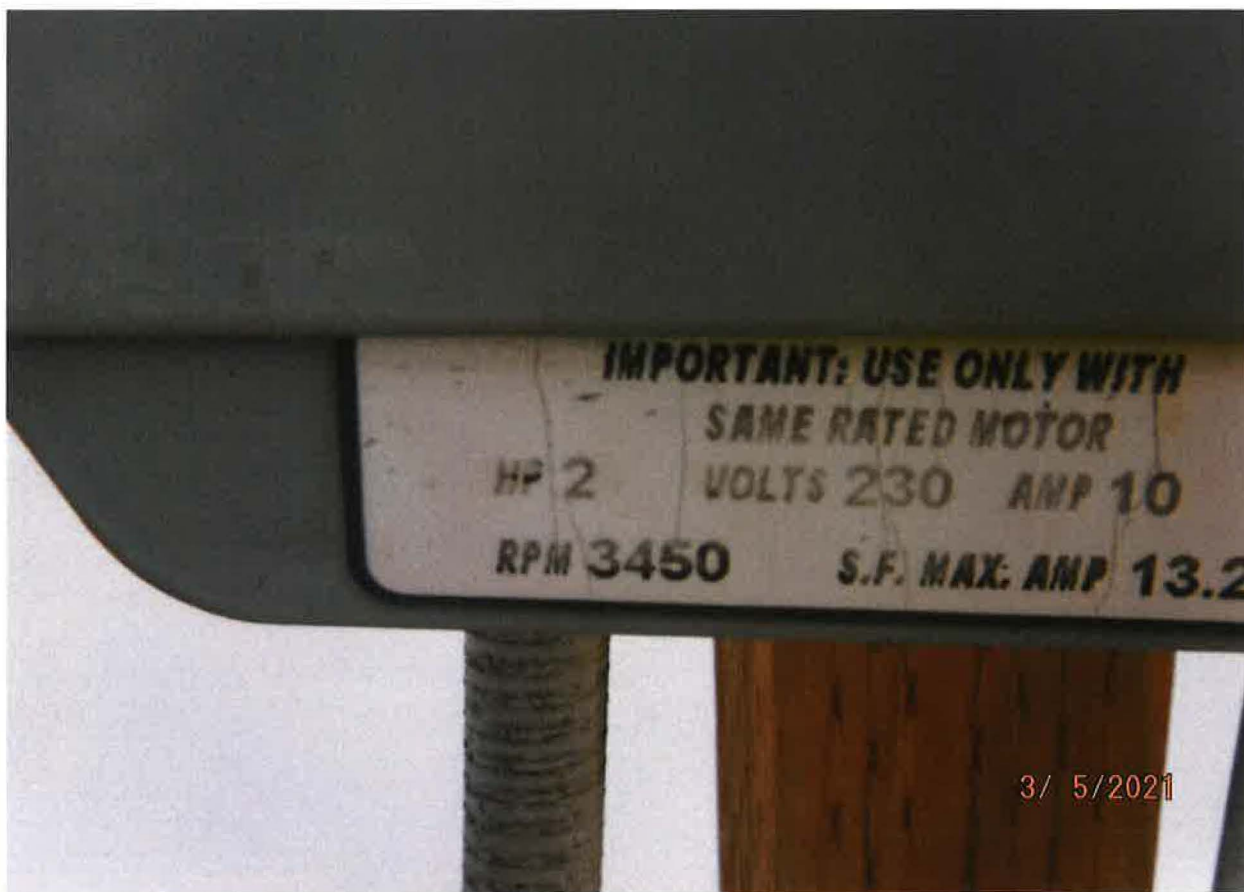
2 HP PUMP MOTOR INSTALLED ON PUMP IN WELL
