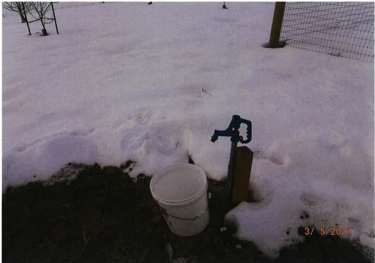
5 GALLON BUCKET FLOW MEASUREMENT TAKEN FROM FROST FREE HYDRANT
