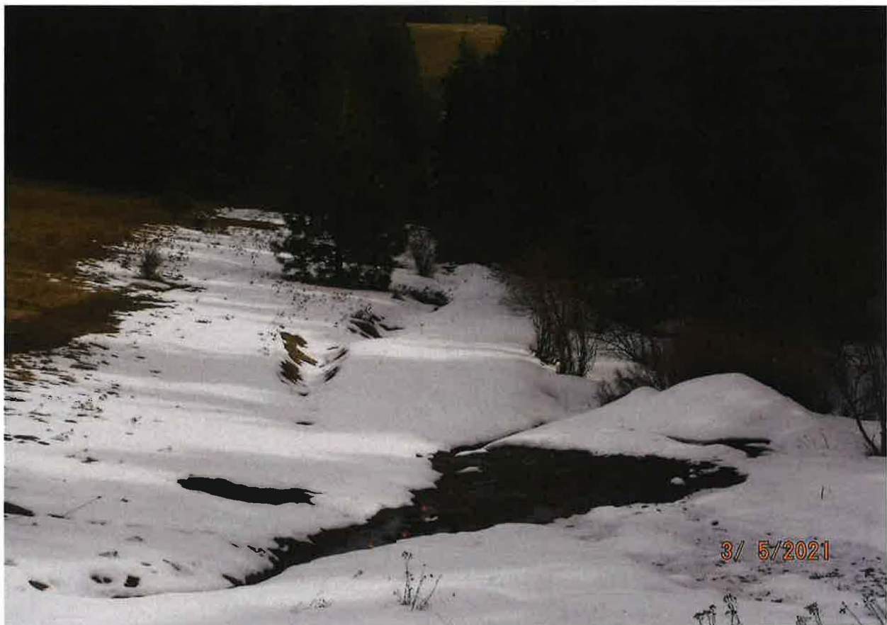
EXIT AREA FOR PRIMARY OVERFLOW DISCHARGE PIPE
