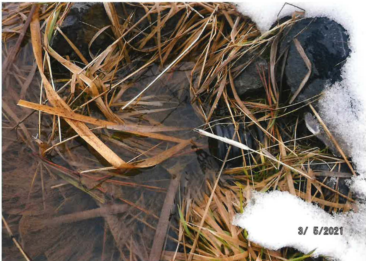
PRIMARY OVERFLOW DISCHARGE FROM POND – 4 INCH CORRUGATED FLEX PIPE
