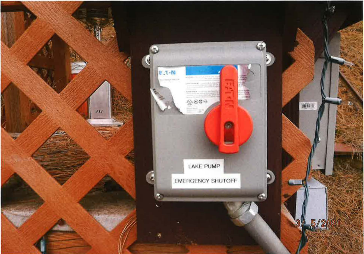
EMERGENCY SHUTOFF VALVE
