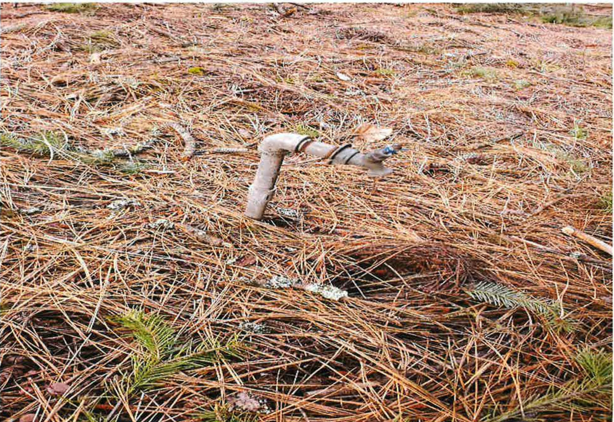
DOMESTIC POU – VACANT LOT – PARCEL No. RP49N04W115005 – STUB-IN AND FROST FREE HYDRANT
