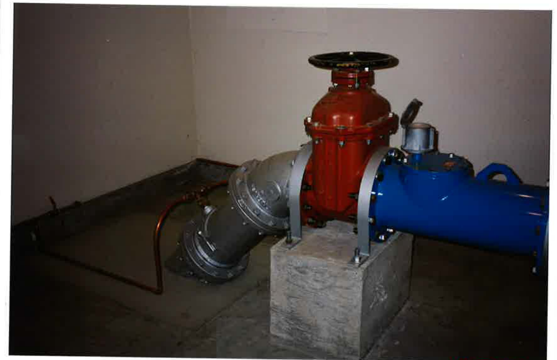
Service line to subdivisions.
