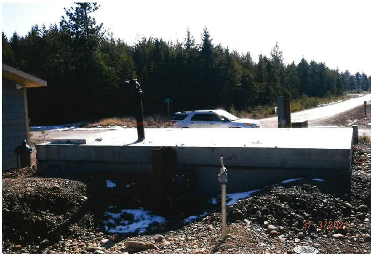
9,000 GAL STORAGE RESERVOIR
